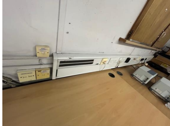
Trunking example to be stripped out
