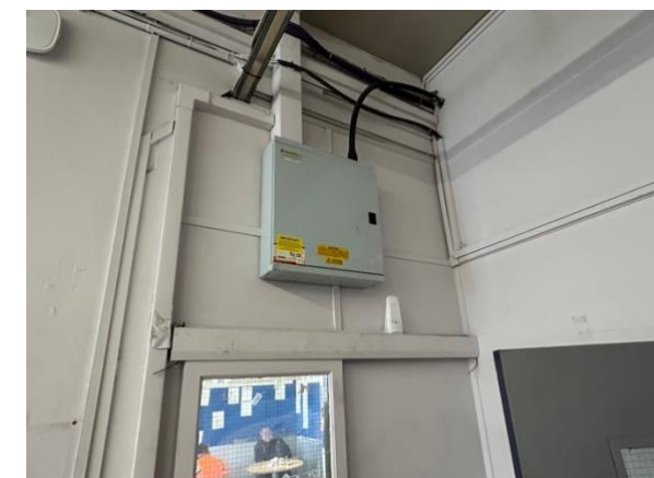
Existing ditribution board to be stripped out
