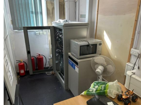
Existing distribution board to be stripped out Data cabinet to remove and replaced with 2no wall mounted cabinets
