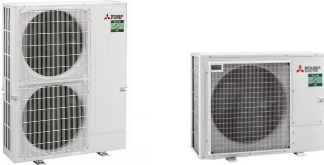
Figure 1-2 (Left) 4no. existing MITSUBISHI ELECTRIC PUZ-ZM250YKA2 and (right) 2no. new PUZ-ZM125YDA units.
