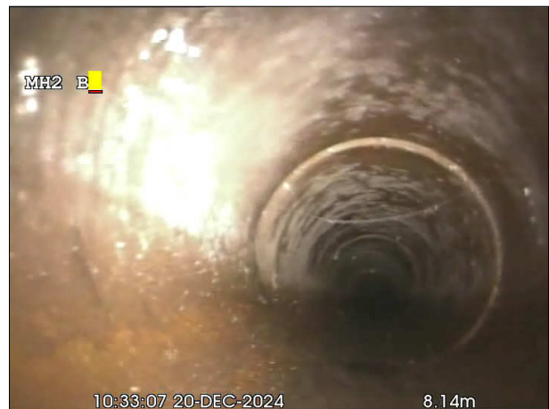
Photo: 55_16a, 00:00:00 8.1m, Joint displaced. Medium
