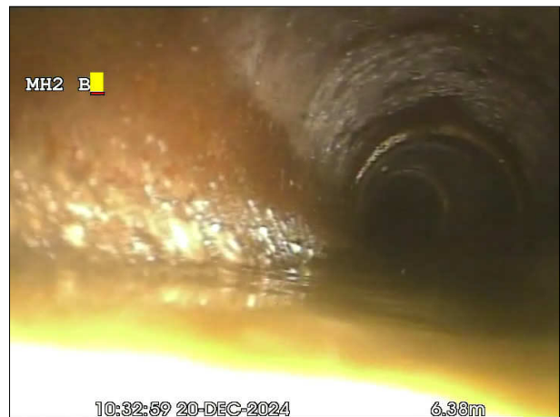
Photo: 54_12a, 00:00:00 6.3m, Joint displaced. Medium
