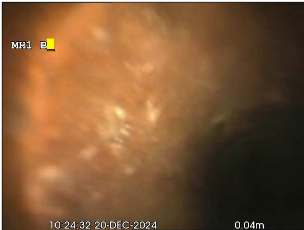
Photo: 53_4a, 00:00:00 0.1m, Line of Sewer deviates right
