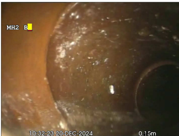
Photo: 5_6a, 00:00:00 0.15m, Line of Sewer deviates right
