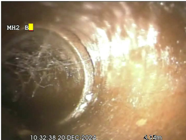
Photo: 5_9a, 00:00:00 4.4m, Line of Sewer deviates left
