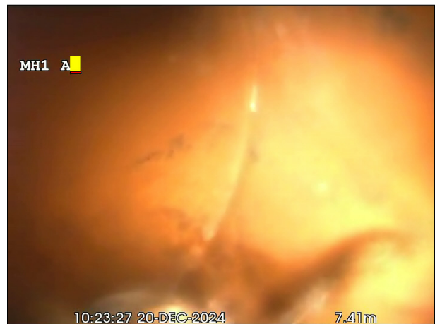
Photo: 20_7a, 00:00:00 7.4m, Line of Sewer deviates up
