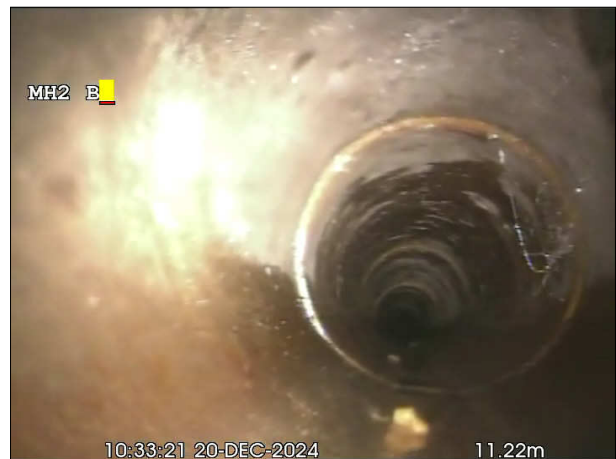
Photo: 57_20a, 00:00:00 11.2m, Joint displaced. Medium
