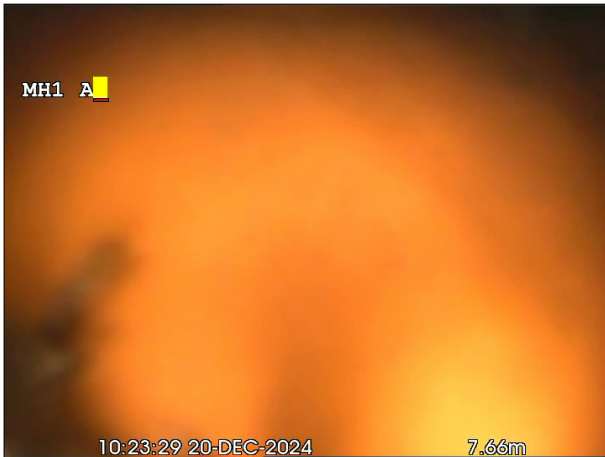
Photo: 22_8a, 00:00:00 7.65m, Debris silt, 15 % cross-sectional area loss, Finish
