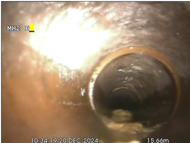
Photo: 60_25a, 00:00:00 15.7m, Joint displaced. Medium,
