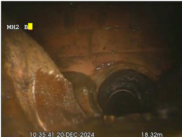
Photo: 5_30a, 00:00:00 18.3m, Debris, 15 % cross-sectional area loss, Finish
