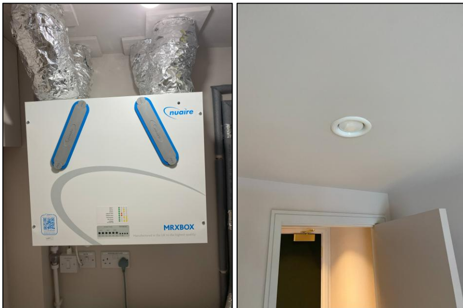
Figure 4.3 - Photographs showing MVHR fan unit and bedroom air supply valve
