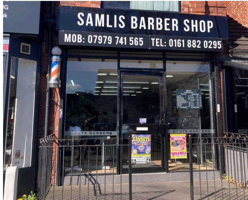
Front Façade in need of repair
