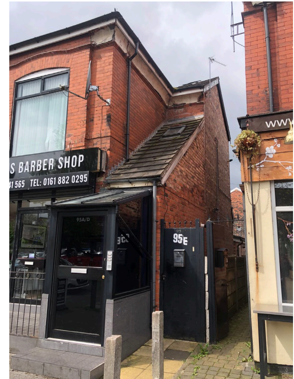
Side walls and roof requires repairs to prevent water egress
