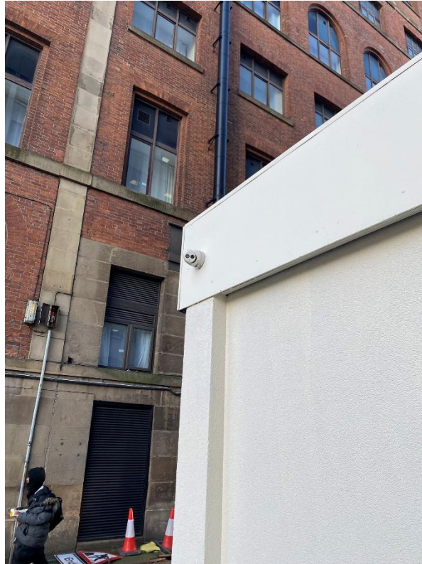
Photograph 7 – Part of External CCTV installation covering whole site
