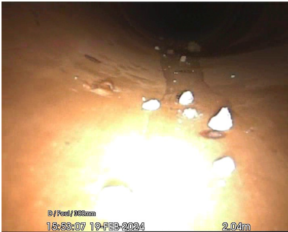
38X_a4c8fb9b-916e-4ed0-ba2d-8d6210d3afb6_20240220_1312_229.jpg, 00:00:07, 2.04 m Settled deposits, coarse, 5% cross-sectional area loss
