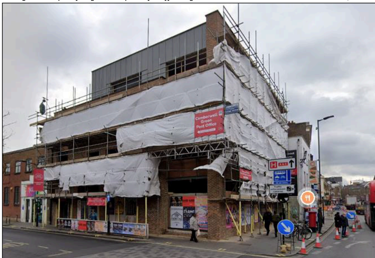
Fig 2: Example of negative impact of scaffolding on the street scene at Camberwell Green, London
