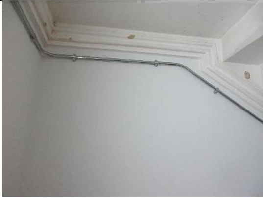
Example of trunking following soffit line
