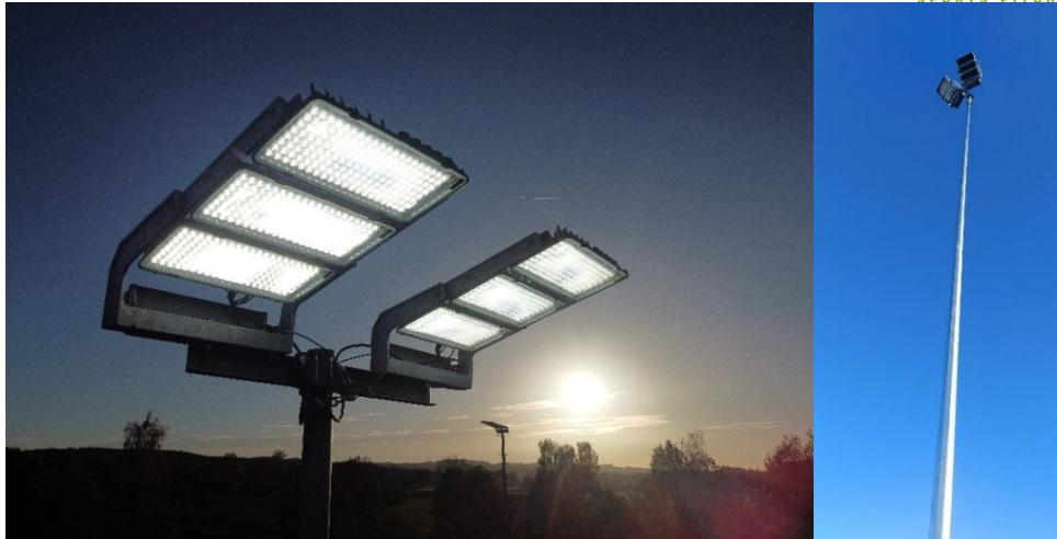
Figure 2 - A Typical Example of Philips Luminaires and Columns
