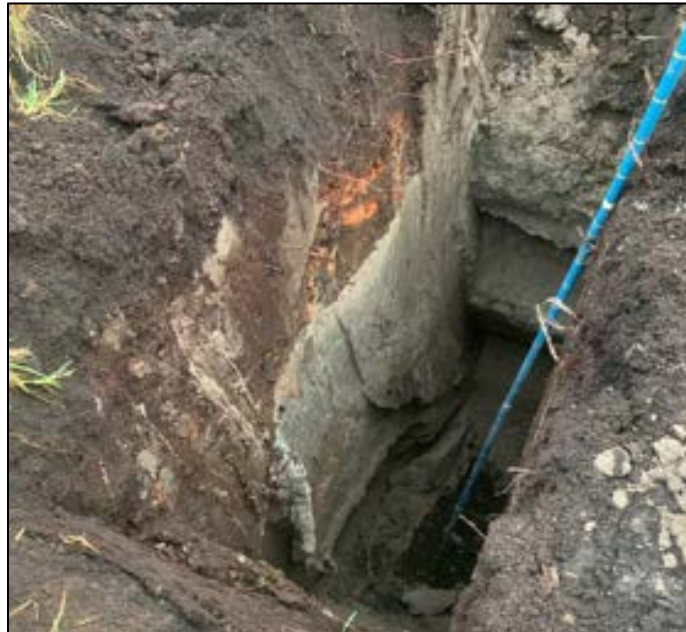
Figure 13: TP09 upon completion showing a collapse of the pit wall within the silt at the base of the pit.
