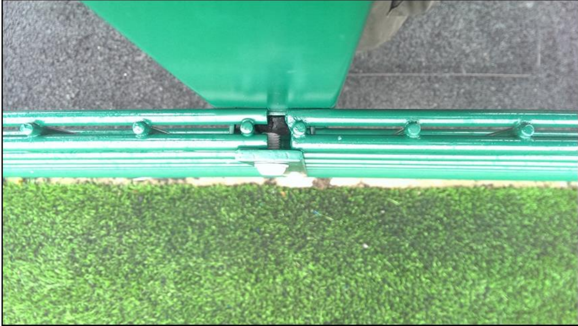
Figure 10: Image Showing Neoprene Isolators
