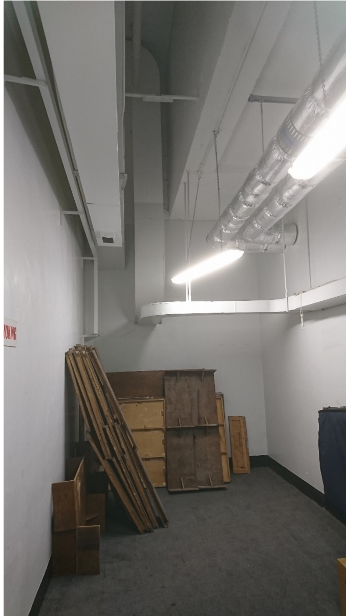
05-27 View of storage cupboard with original components of the M&E system.
