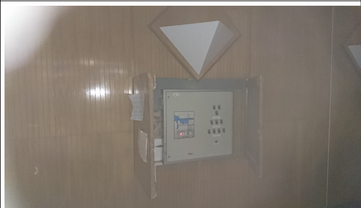
05-21 View of the built in electrical controls to lighting within the wall panelling.
