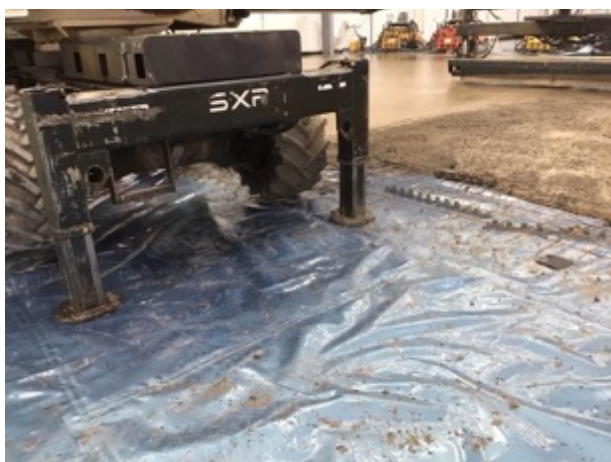
Plant keeping off the mesh over the membrane
