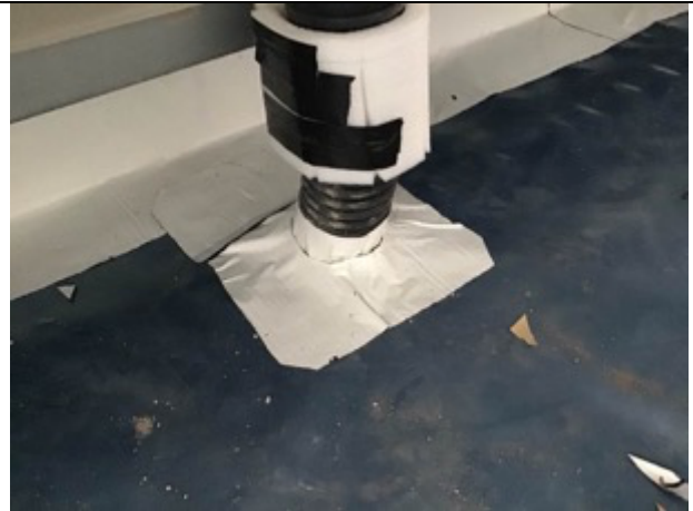
Unit 2 retro fit detailing and sealed pipe penetration
