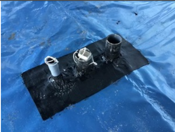
Unit 3 sealed pipe penetrations
