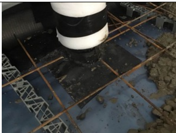
Sealed pipe penetration
