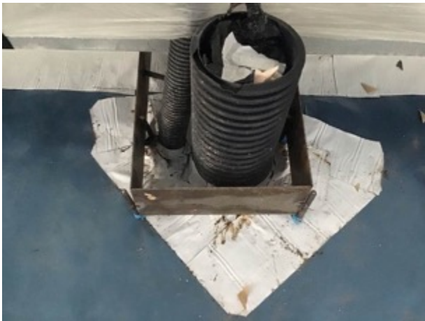
Unit 3 sealed pipe penetrations
