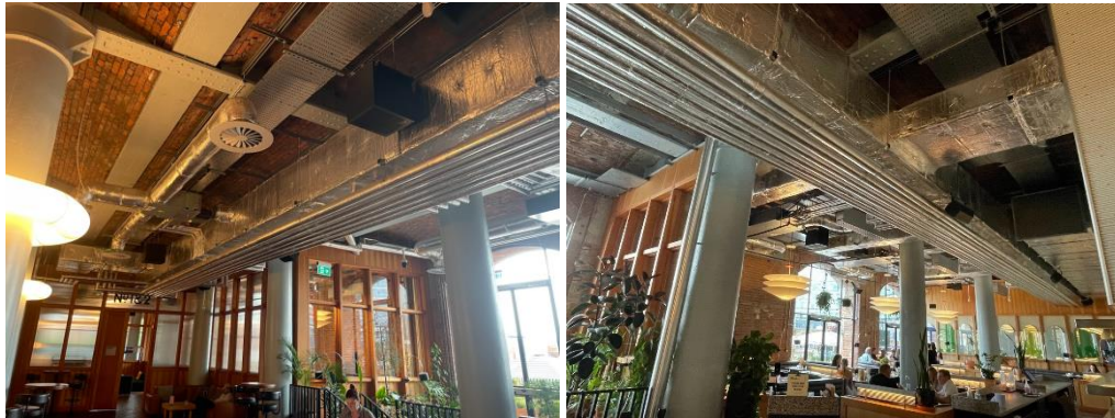
Figure 4.4: View of existing mechanical plant and ducting with Ducie Street Warehouse
