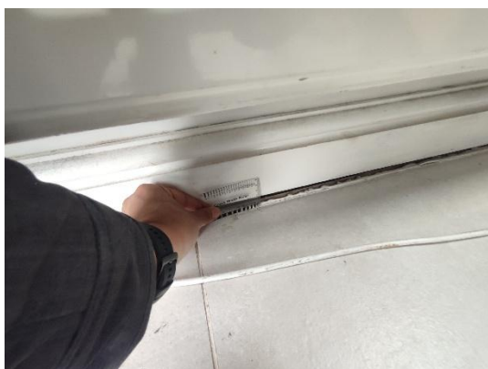
Photo 24 – 20mm gap between flooring and skirting boards, the presence of sealant on the tiles is indicative that this has occurred in the recent past.
