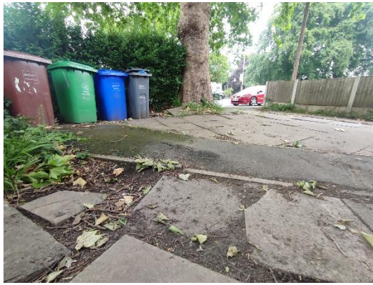
Photo 5 – View of raised flagstones and localised undulations in the front garden
