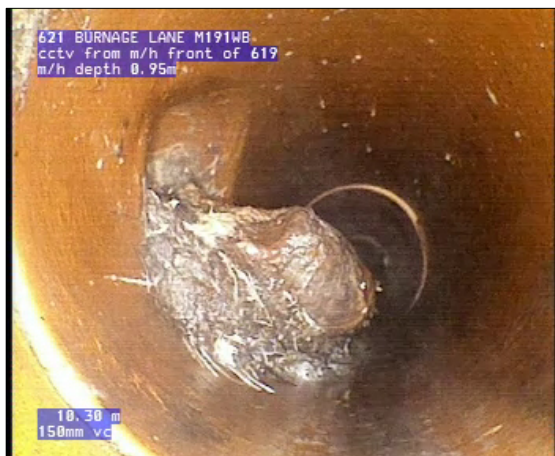
Photo: 5_5_44_A.jpg, 00:01:24 10.3m, Junction, at 10 o'clock, diameter 100mm Remarks: Full of roots
