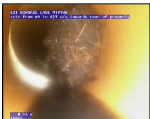
Photo 12 – 50% blockage to the side elevation (Ch. 0.14m)
