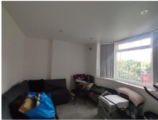
Photo 17 – View of the room overlooking the front garden, cracks observed on walls perpendicular to front elevation wall and bay window construction measured/observed to incline slightly
