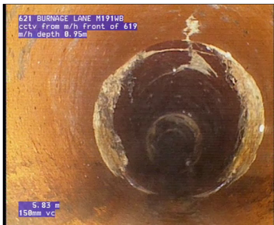
Photo: 5_5_40_A.jpg, 00:00:49 5.83m, Fracture, circumferential at joint, from 11 to 1 o'clock
