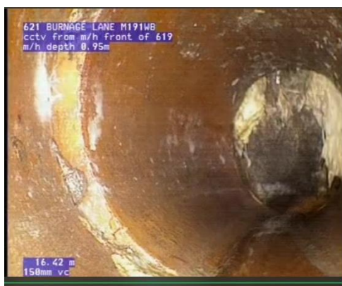
Photo 11 – 95% blockage at the front of the property (Ch. 16.54m, see drainage report)
