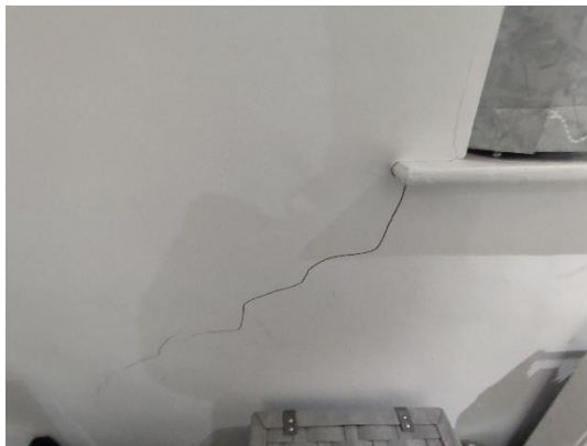
Photo 27 – View of the 2mm wide diagonal stepped crack to the bottom left corner of the window
