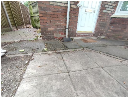
Photo 6 – Undulations observed in the surfacing adjacent to the front and side elevations. The client highlighted that the drains were previously inspected and significant root ingress was observed.
