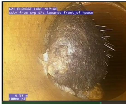
Photo 10 – 50% blockage observed in the drain pipe at the front of the property (Ch. 6.59m)
