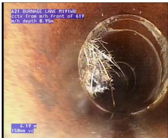
Photo: 5_5_36_A.jpg, 00:00:32 4.19m, Roots, mass at joint, 10% cross-sectional area loss
