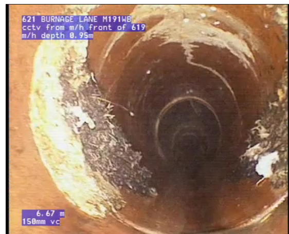
Photo: 5_5_41_A.jpg, 00:00:53 6.67m, Attached deposits, encrustation at joint, from 7 to 5 o'clock, 10% cross-sectional area loss
