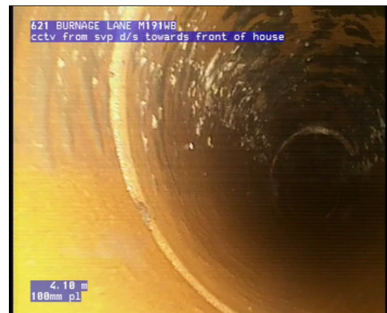
Photo: 1_1_10_A.jpg, 00:00:46 4.1m, Attached deposits, grease, from 9 to 3 o'clock, 5% cross-sectional area loss, Start
