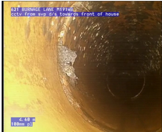
Photo: 1_1_11_A.jpg, 00:00:49 4.6m, Roots, fine at joint
