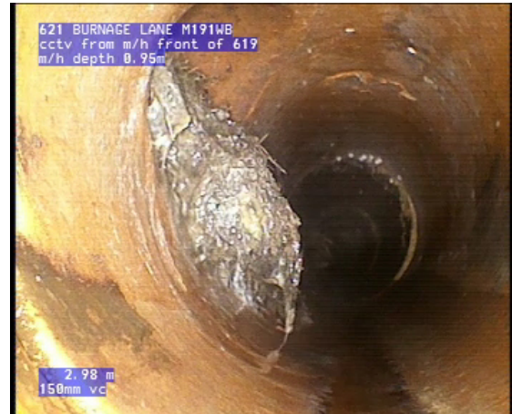
Photo: 5_5_35_A.jpg, 00:00:21 2.98m, Junction, at 11 o'clock, diameter 100mm Remarks: Roots coming out from junction
