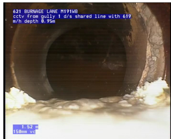
Photo: 3_3_25_A.jpg, 00:00:32 1.52m, Joint displaced, large
