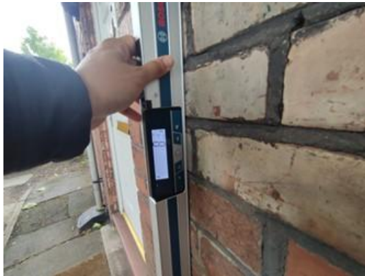
Photo 14 – Inclination of front elevation wall measured having an incline of up to 8mm per meter
