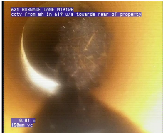
Photo: 6_6_52_A.jpg, 00:00:05 0.01m, Roots, mass at joint, 50% cross-sectional area loss
