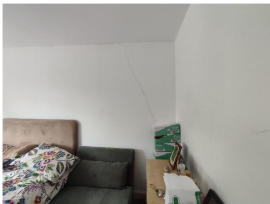
Photo 36 – Diagonal cracks observed on the party wall indicative of slight movements of the foundations potentially affecting both properties
