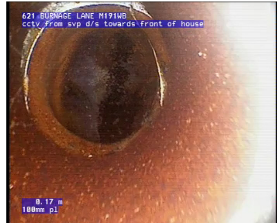
Photo: 1_1_5_A.jpg, 00:00:13 0.08m, Fracture, circumferential at joint, from 1 to 4 o'clock
