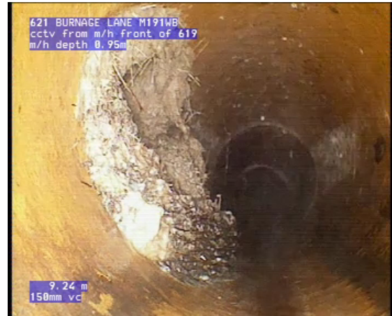
Photo: 5_5_43_A.jpg, 00:01:12 9.24m, Junction, at 10 o'clock, diameter 100mm Remarks: Full of Roots
