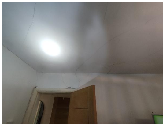
Photo 19 – Widespread diagonal cracks (<1mm wide), indicative of ongoing movements
