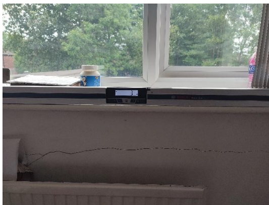
Photo 31 – Horizontal cracks beneath the window and inclinations of 3mm per metre observed on the window sill
