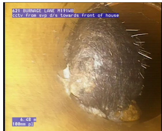
Photo: 1_1_14_A.jpg, 00:01:07 6.48m, Roots, mass at joint, 50% cross-sectional area loss
