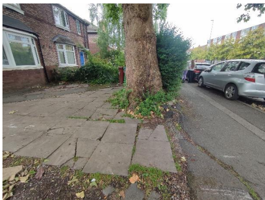
Photo 3 – View of base of tree and damage to concrete flagstones and surfacing of public footway
