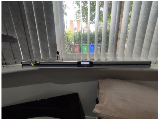
Photo 18 – Horizontal checks of the bay window area indicate inclinations of 7mm per meter, cracks also noted on the walls perpendicular to this wall
