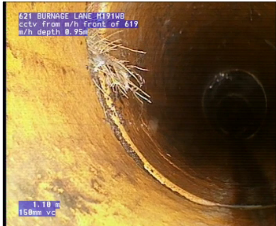
Photo: 5_5_34_A.jpg, 00:00:09 0.99m, Roots, fine at joint
