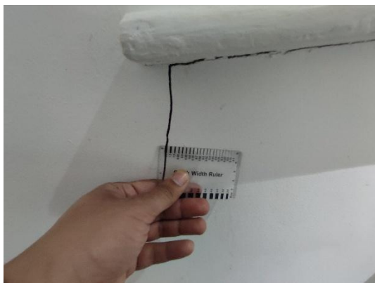
Photo 28 – Crack measured as 2mm wide
