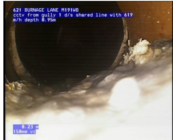
Photo: 3_3_23_A.jpg, 00:00:19 0.14m, Joint displaced, large
