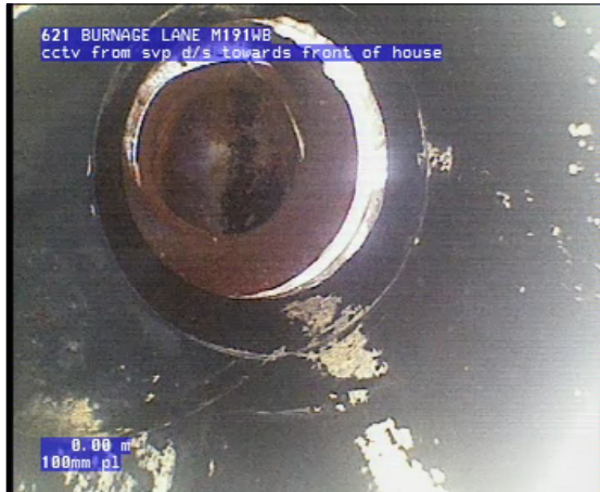
Photo: 1_1_4_A.jpg, 00:00:01 0m, Fracture, circumferential at joint, from 7 to 5 o'clock
