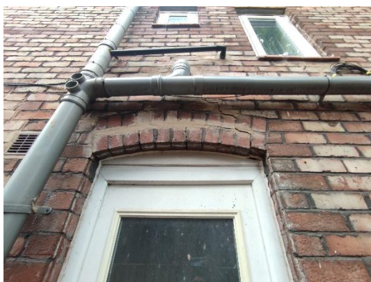
Photo 16 – Diagonal stepped cracking noted above the ground-floor segmental arch lintel (cracking to right).
