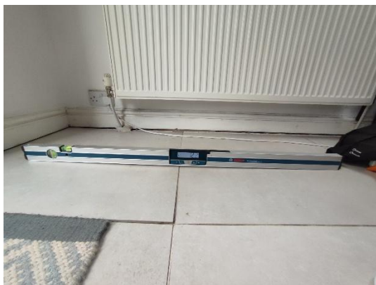
Photo 23 – Floor dropping in areas, 20mm gap noted between flooring and skirting boards, horizontal inclinations of up to 12mm per meter recorded.
