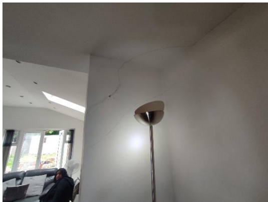
Photo 22 – Diagonal cracks extending to party wall with neighbouring property
