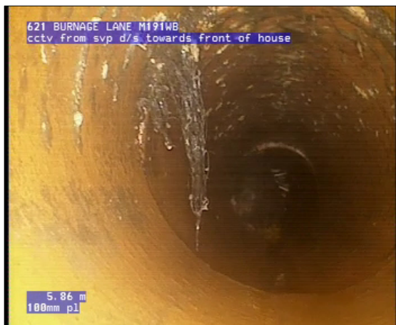
Photo: 1_1_13_A.jpg, 00:00:59 5.86m, Roots, fine at joint
