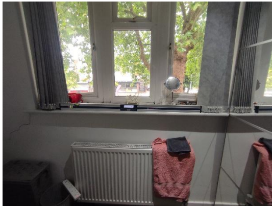
Photo 26 – Close up of bay window. Slight inclination of 4mm per metre observed. 2mm wide diagonal stepped crack located at the bottom corner of the window. Further diagonal crack observed behind the wardrobe at the top right of this window.
