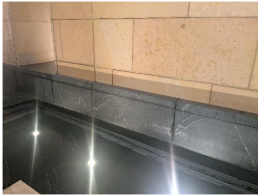
Figure 14: 1990s water feature – reportedly non-functional/prone to leaking.
