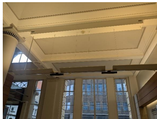
Figure 17: Suspended lighting in reception area.
