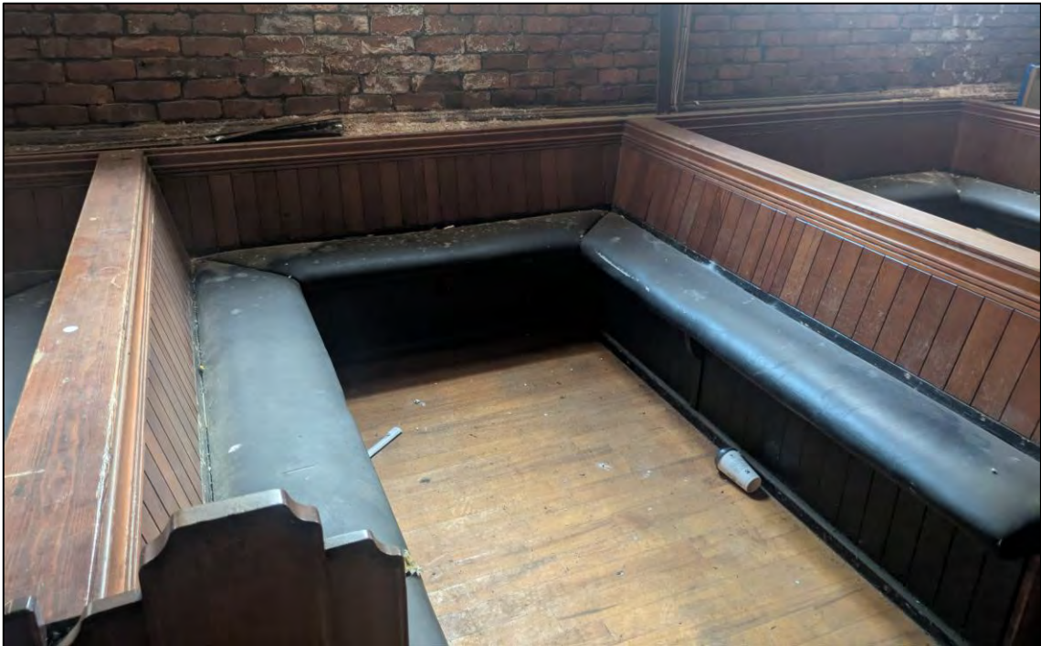
Plate 6: Historic Pews and Joinery and Evidence of Efflorescence on Brickwork
