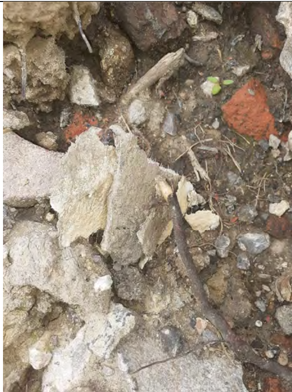
Figure 5: AIB encountered within boiler room
