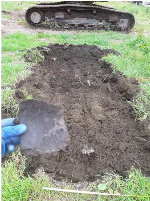
Figure 4: Suspect asbestos bitumen pipe within contaminated soils
