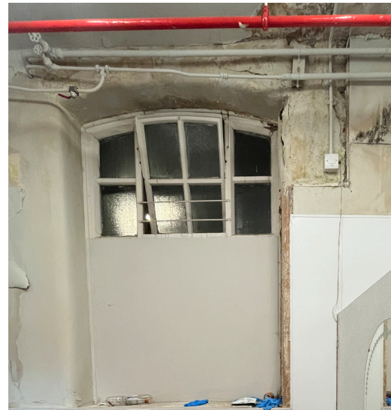
Boarded up lower section of WC GF.10 window to be removed and film applied to lower panes to provide privacy as below
