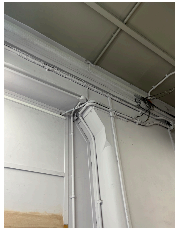
Extensive services fixed to wall detract from the building form
