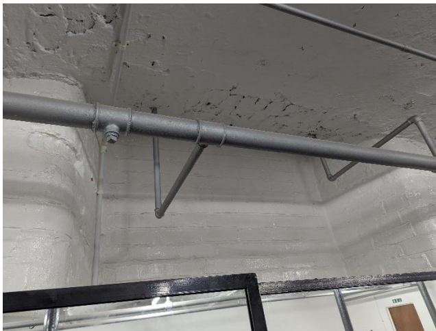
Supply To First Floor Radiators
