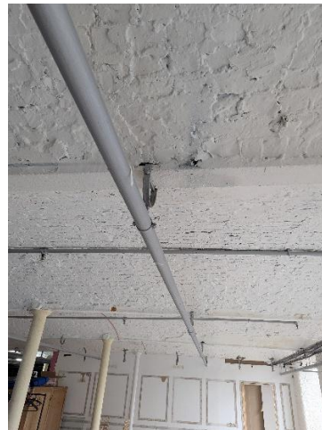
One Of Four Parallel Pipes
