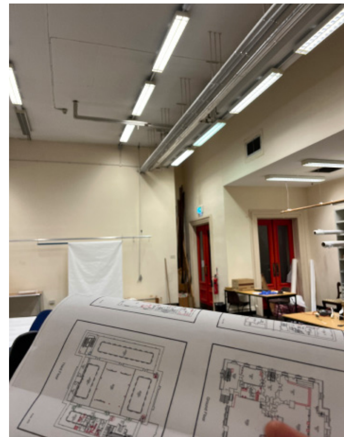
Figure 6 Level 01 Archive Store, these areas have plain, painted exposed ceilings and walls. There are exposed services present, the new fire alarm will re-used existing metal cable trays, cable runs, fixing points and detector head positions.
