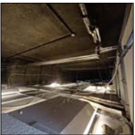
2 - Above Frances Dean Room, form small bulkhead to avoid Pipe work.
