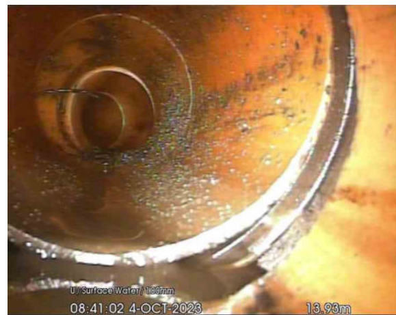
MH3 US ACO_13-93m_084102.jpg, 00:01:23, 13.93 m Joint displaced, large
