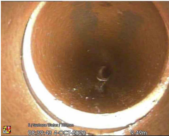
MH3 US ACO_9-49m_083943.jpg, 00:00:41, 9.49 m Joint displaced, medium
