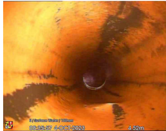
MH3 US RWP_4-52m_083557.jpg, 00:00:25, 4.52 m Deformed sewer or drain, 10%
