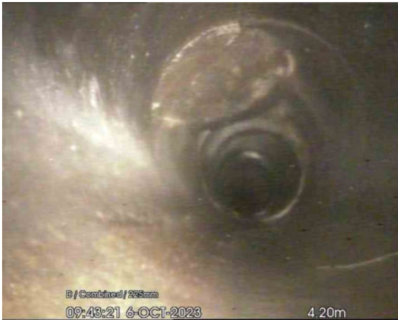
MH C1 DS_4-20m_094321.jpg, 00:00:22, 4.20 m Hole in drain or sewer from 9 o'clock to 2 o'clock, POOR REPAIR
