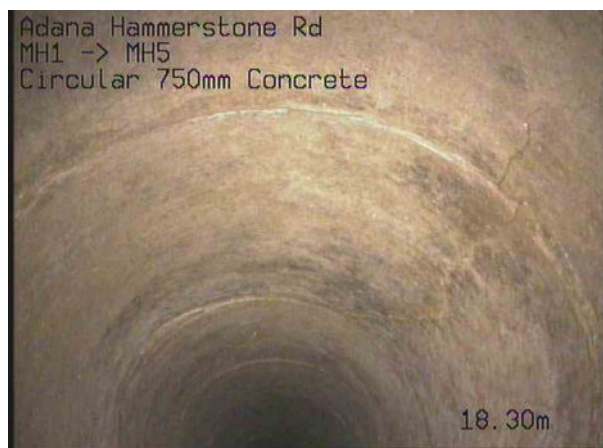
MH1X_c2594daa-fcaf-402d-bd67-0043181de174_20230929_082633_141.jpg, 00:03:37, 18.30 m Fracture, longitudinal at 2 o'clock, start
