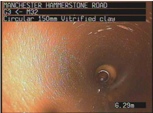
G3X_0aa1f7fa-6cd4-4596-b480-e012c28a25d0_20230822_14 5216_936.jpg, 00:00:42, 6.29 m Surface damage, spalling from 10 o'clock to 2 o'clock
