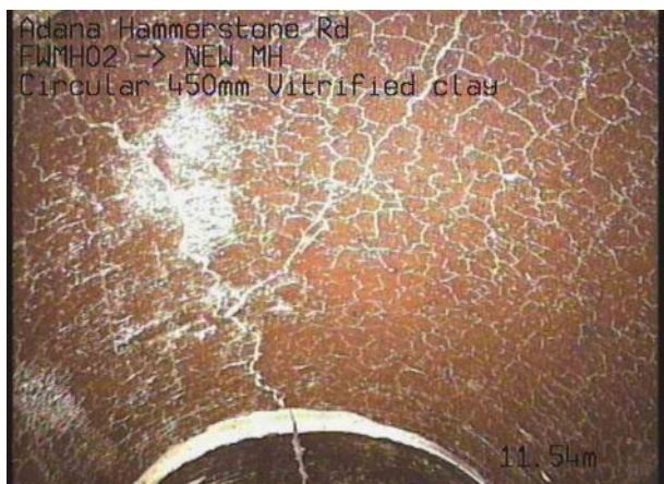
FWMH02X_633f7784-7216-4371-80bf-317db178d39e_20230929_125002_555.jpg, 00:05:27, 11.54 m Fracture, longitudinal at 12 o'clock, start
