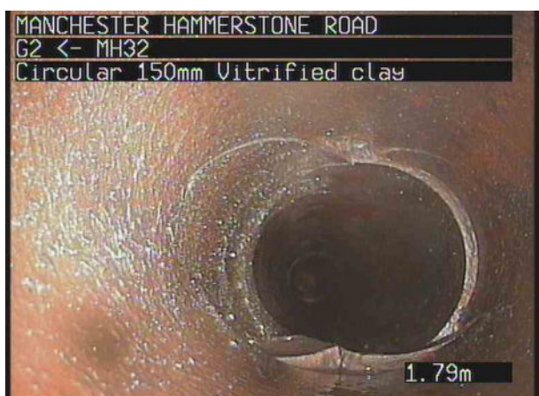
G2X_747da227-0512-4bbe-84f2-efa2331e3276_20230822_14 4655_798.jpg, 00:01:08, 2.30 m Deformed sewer or drain, 10%
