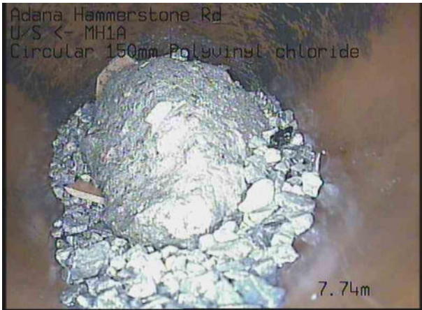
U_SX_551ced77-9085-490f-9a3d-03c1825fe094_20231002_1 11536_088.jpg, 00:01:23, 7.74 m Collapsed drain or sewer, 95% cross-sectional area loss
