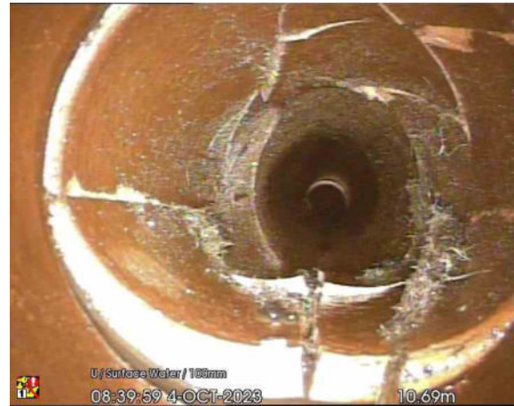
MH3 US ACO_10-69m_083959.jpg, 00:00:48, 10.69 m Fractures, multiple at 12 o'clock
