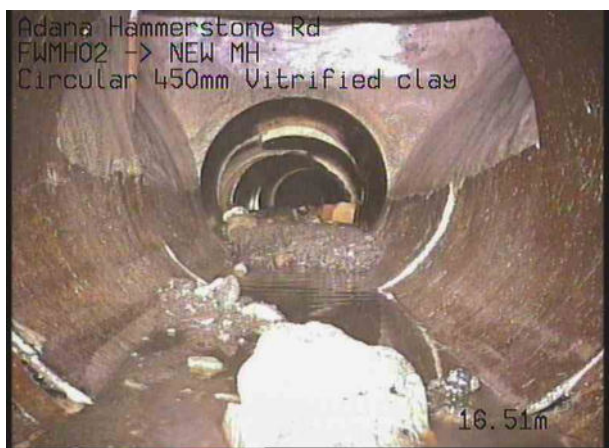
FWMH02X_88bea82c-ac8f-4bd6-ad0a-3f201e129369_20230929_125210_984.jpg, 00:07:37, 16.51 m Other obstacles, brick or masonry in invert at joint from 5 o'clock to 6 o'clock, 10% cross-sectional area loss
