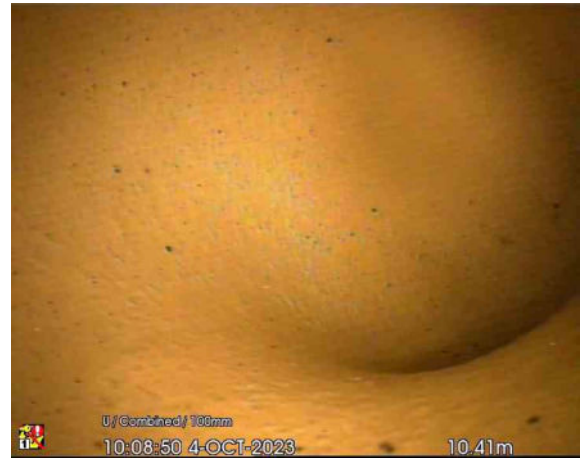
MH24 US_10-41m_100850.jpg, 00:01:26, 10.41 m Survey abandoned, UNABLE TO PASS BENDS
