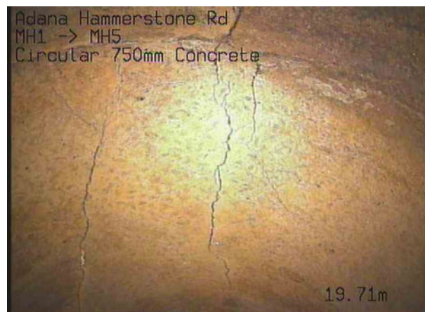
MH1X_56c66650-3221-4101-b6ba-7d3f042609b4_20230929_082729_854.jpg, 00:04:34, 19.71 m Fractures, multiple from 11 o'clock to 2 o'clock
