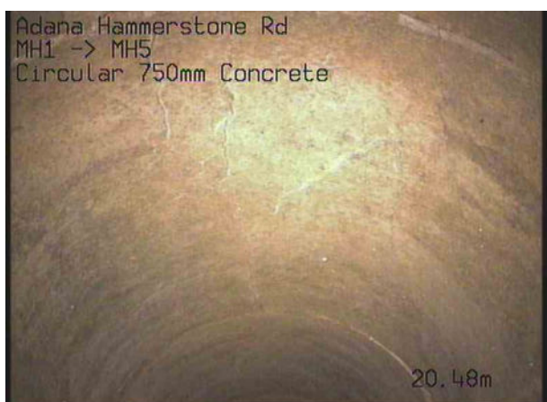
MH1X_e097ea5e-e366-4a2c-9436-68de88a165e2_20230929_082822_672.jpg, 00:05:06, 20.48 m Fractures, multiple from 12 o'clock to 12 o'clock, start
