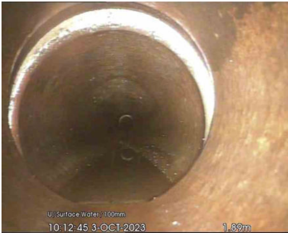
MH19 US GULLY_1-89m_101245.jpg, 00:00:16, 1.89 m Joint displaced, medium
