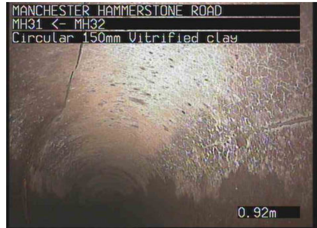
MH31X_a7e1bd3b-4274-4a7a-8eac-753dbce24893_20230822_142250_429.jpg, 00:00:24, 0.90 m Fracture, longitudinal at joint at 11 o'clock
