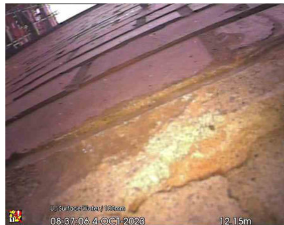
MH3 US RWP_12-15m_083706.jpg, 00:01:02, 12.15 m Survey abandoned, RWP MISSING OFF WALL
