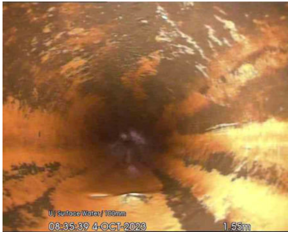
MH3 US RWP_1-55m_083539.jpg, 00:00:12, 1.55 m Deformed sewer or drain, 15%
