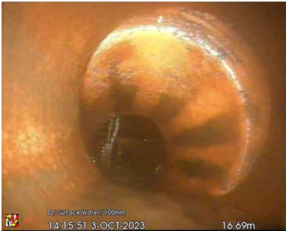
MH4 DS MH5_16-69m_141551.jpg, 00:01:10, 16.69 m Joint displaced, medium
