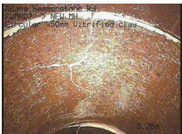
FWMH02X_d67fa18a-261f-42cc-b472-823572ada9df_20230929_124648_735.jpg, 00:02:12, 3.26 m Fracture, longitudinal at 12 o'clock, start
