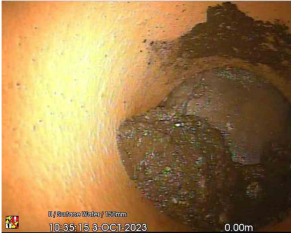
MH26 US_0-00m_103515.jpg, 00:00:02, 0.00 m General remark, CAPPED
