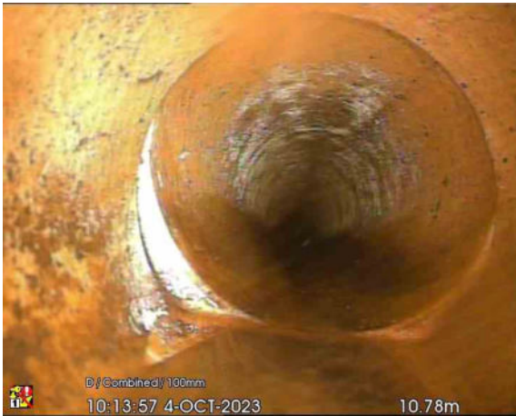
MH24 DS_10-78m_101357.jpg, 00:00:41, 10.78 m Joint displaced, medium
