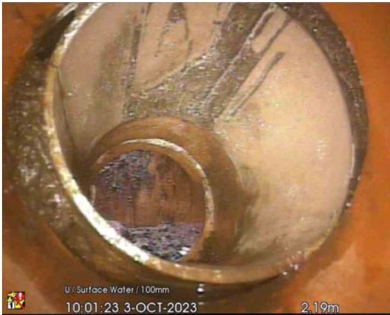
MH18 US GULLY_2-19m_100123.jpg, 00:00:14, 2.19 m Joint displaced, large
