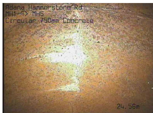
MH1X_3d9dbc05-6e24-48b4-bd28-cb39d0947a73_20230929_082952_988.jpg, 00:06:57, 24.56 m Fracture, longitudinal at 12 o'clock, start
