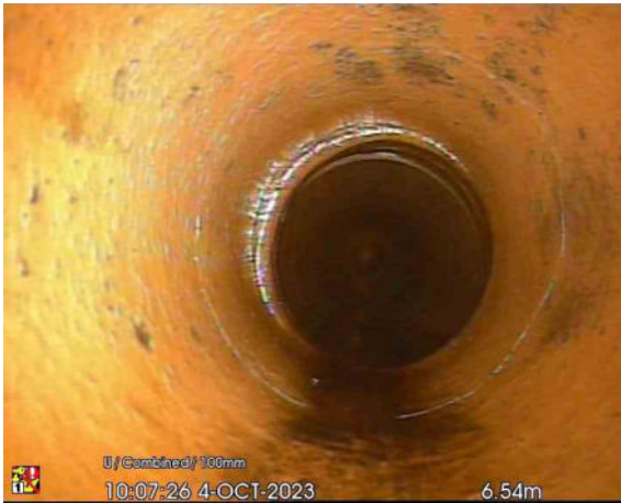
MH24 US_6-54m_100726.jpg, 00:00:35, 6.54 m Fracture, circumferential at joint at 12 o'clock
