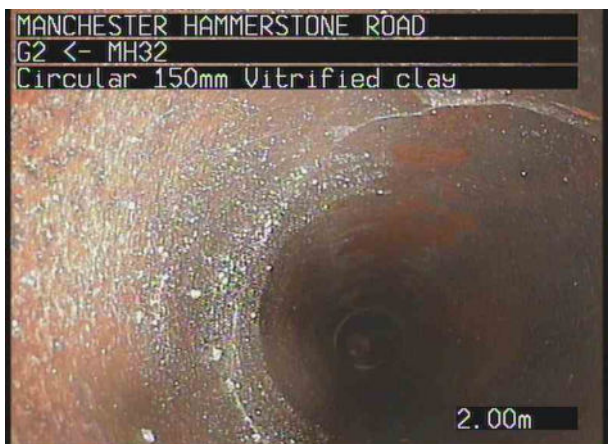
G2X_d3ff5865-e93a-4ec7-a84c-383277f4871d_20230822_14 4547_320.jpg, 00:00:26, 2.00 m Fracture, circumferential at joint from 12 o'clock to 12 o'clock, FROM HOLE
