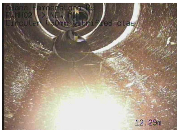
FWMH02X_f3b58675-fd07-4717-8b15-d7f2aa510cb6_20230929_125036_729.jpg, 00:06:02, 12.29 m Fracture, longitudinal at 6 o'clock
