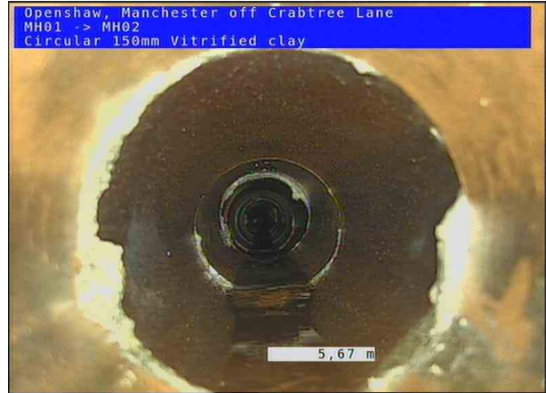
MH01X_bcc62be9-2ae3-41de-a47b-d78b27a57ecd_20240604_105731_164.jpg, 00:02:24, 5.67 m Survey abandoned, ENCRUSTATION, SCALE 15%
