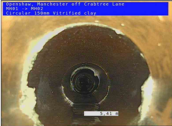
MH01X_8f5b6865-c3ca-404c-b066-ae3b44a98915_20240604_105605_389.jpg, 00:01:30, 5.41 m Attached deposits, encrustation at joint from 7 o'clock to 10 o'clock, 15% cross-sectional area loss
