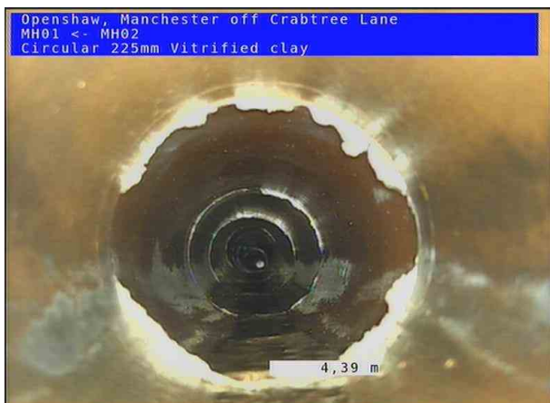
MH01X_707ffdc7-f186-42af-b54b-9dd9e84b2793_20240604_110601_419.jpg, 00:00:57, 4.39 m Attached deposits, encrustation at joint from 12 o'clock to 12 o'clock, 15% cross-sectional area loss
