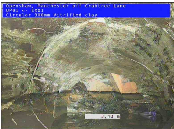
UP01X_5bcc3133-3077-4964-8679-81de97dabb64_20240604_093536_827.jpg, 00:02:05, 3.43 m Water level, 40% of the vertical dimension
