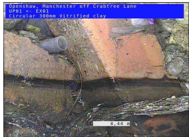
UP01X_d248183a-bef2-40cf-9ece-b15934de1512_20240604_093654_879.jpg, 00:03:10, 4.44 m Collapsed drain or sewer, 100%
