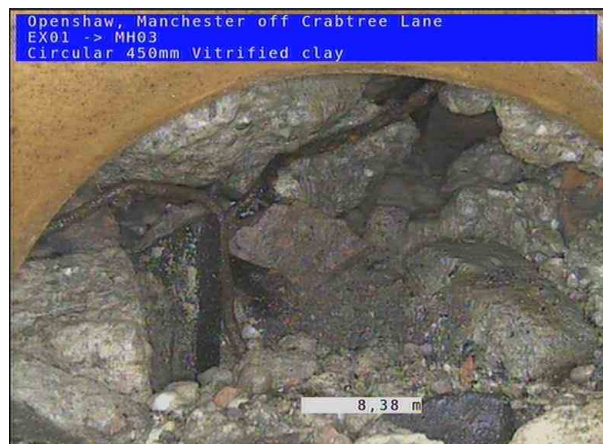
EX01X_91472800-c21d-4980-93ed-87aae1a343d1_20240604_102627_716.jpg, 00:02:32, 8.38 m Survey abandoned, COLLAPSED PIPE
