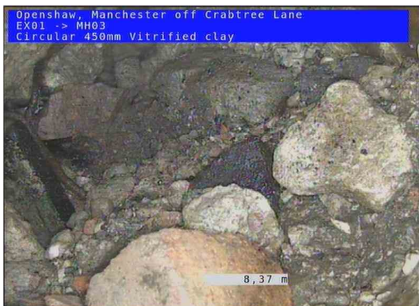
EX01X_9ded35e4-c10f-454f-a2a1-fa3eb9e97bb7_20240604_102543_161.jpg, 00:01:44, 8.37 m Collapsed drain or sewer, 100%
