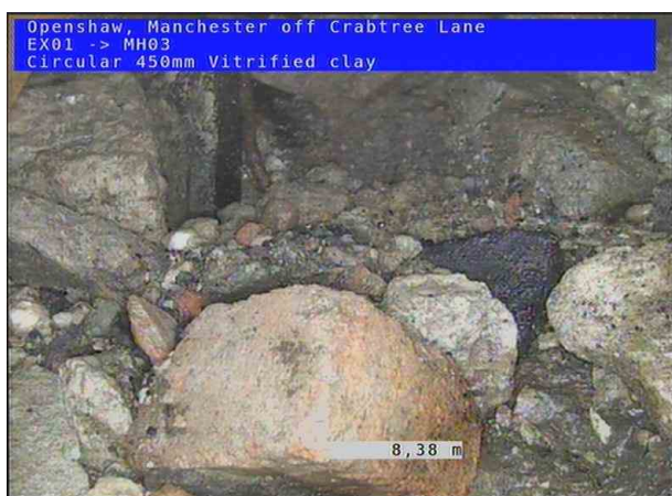
EX01X_c373c107-d9d9-4575-a5f7-a1e859cbf025_20240604_102632_009.jpg, 00:02:32, 8.38 m Survey abandoned, COLLAPSED PIPE
