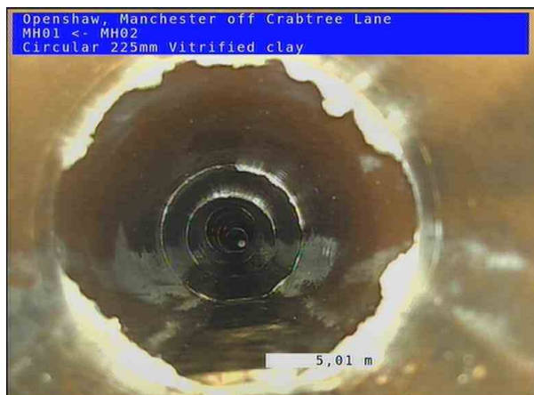
MH01X_684ee632-ca36-4d4a-974c-0a5df5008eea_20240604_110802_901.jpg, 00:02:17, 5.01 m Survey abandoned, ENCRUSTATION, SCALE 15%
