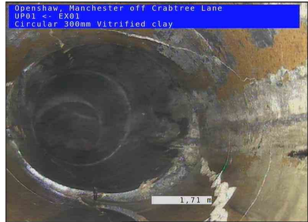
UP01X_4179f33c-7a94-48cf-8a82-e2556515ddb4_20240604_093351_814.jpg, 00:01:10, 1.71 m Fractures, multiple from 12 o'clock to 12 o'clock, start
