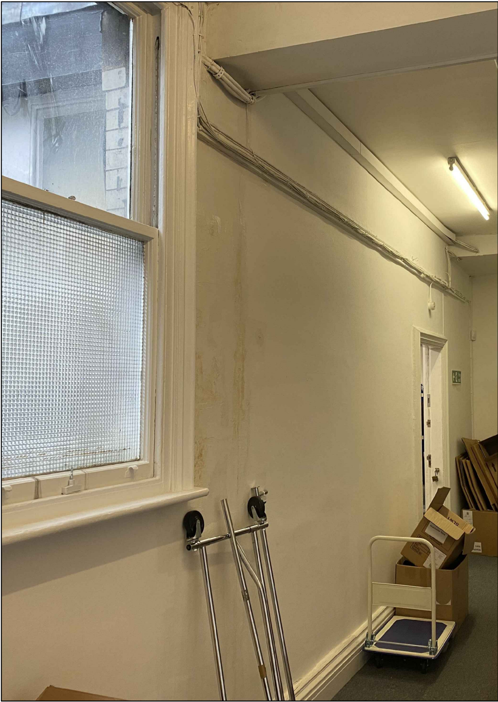
EXISTING ELECTRICAL DISTRIBUTION PHOTO 'B'
