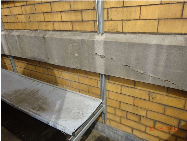
Plate 4: View of cracked Portland stone banding to north elevation parapet
