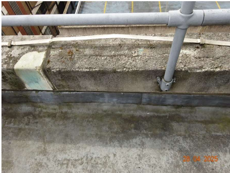
Plate 5: Poor condition of mortar repair to top of south elevation parapet
