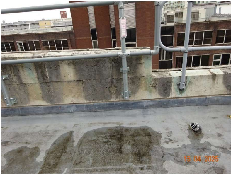
Plate 6: Redundant fixing holes and failed pointing to stone parapets
