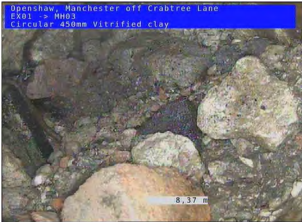
EX01X_9ded35e4-c10f-454f-a2a1-fa3eb9e97bb7_20240604_102543_161.jpg, 00:01:44, 8.37 m Collapsed drain or sewer, 100%
