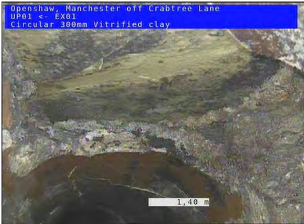
UP01X_0ebc5ec2-7073-45f7-8403-21ec87af57ab_20240604_093311_873.jpg, 00:00:51, 1.40 m Hole in drain or sewer from 11 o'clock to 1 o'clock, POSSIBLE REPAIR
