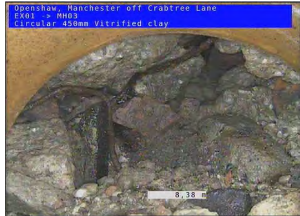
EX01X_91472800-c21d-4980-93ed-87aae1a343d1_20240604_102627_716.jpg, 00:02:32, 8.38 m Survey abandoned, COLLAPSED PIPE
