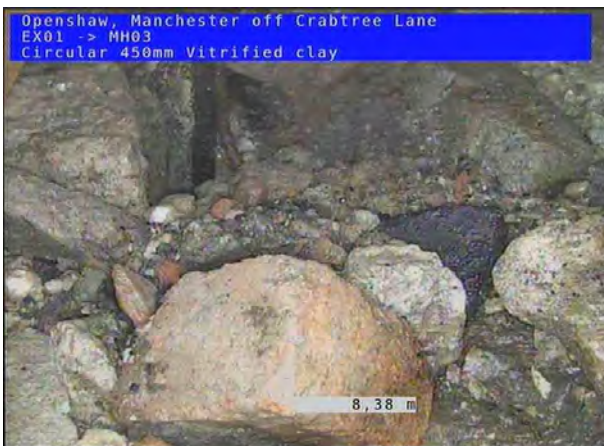
EX01X_c373c107-d9d9-4575-a5f7-a1e859cbf025_20240604_102632_009.jpg, 00:02:32, 8.38 m Survey abandoned, COLLAPSED PIPE
