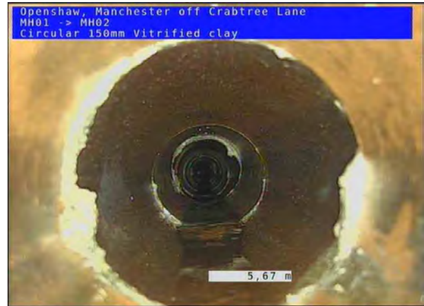
MH01X_bcc62be9-2ae3-41de-a47b-d78b27a57ecd_20240604_105731_164.jpg, 00:02:24, 5.67 m Survey abandoned, ENCRUSTATION, SCALE 15%
