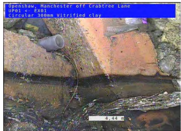
UP01X_d248183a-bef2-40cf-9ece-b15934de1512_20240604_093654_879.jpg, 00:03:10, 4.44 m Collapsed drain or sewer, 100%
