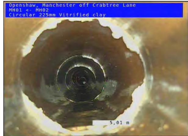
MH01X_684ee632-ca36-4d4a-974c-0a5df5008eea_20240604_110802_901.jpg, 00:02:17, 5.01 m Survey abandoned, ENCRUSTATION, SCALE 15%
