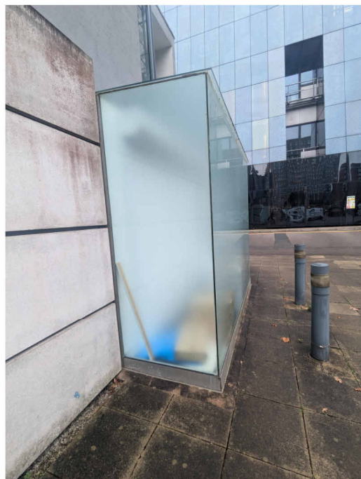
Existing concrete cladding panels are weathered.
