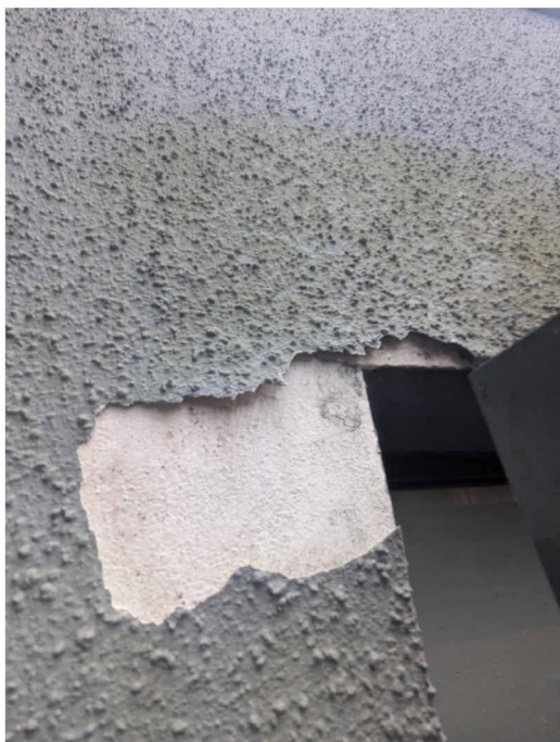
Existing through-coloured render is weathered, with cracking and areas of flaking paint / coatings.
