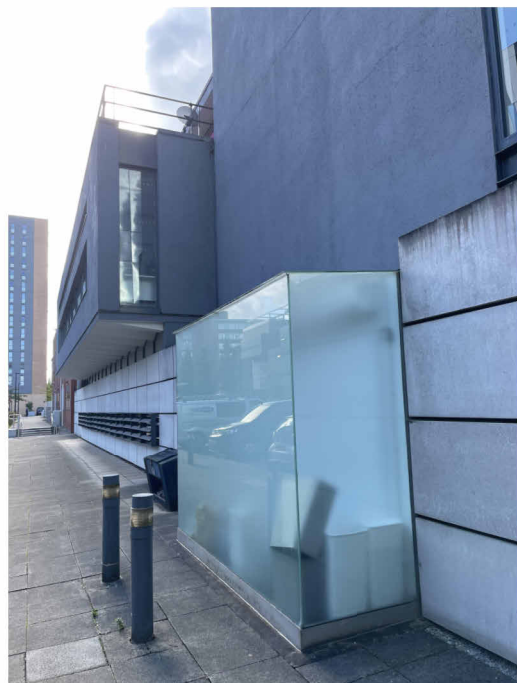
Water ingress to existing planar glazing.
