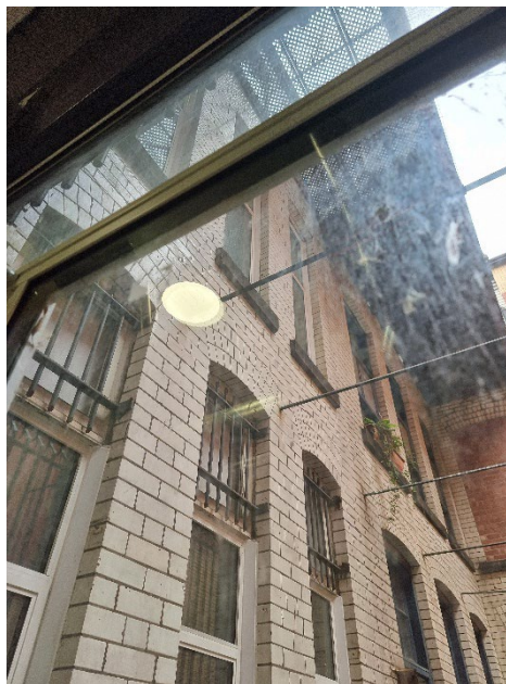
Photograph 7 - View from first floor stairwell window looking up showing the sealed PVCu window units to the apartments and the underside of the decking above.
