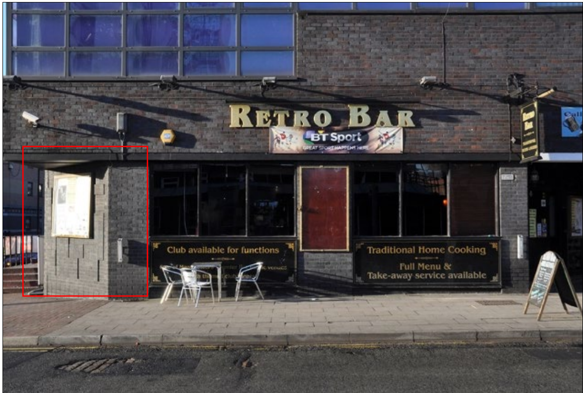
Figure 10: Charles Street Car Park (east elevation, centre). Closeup view of Retro Bar. Original panels to ground floor are lost, and original windows above have been replaced with modern. Note, the geometric mosaic to the SE corner (outlined in red).
