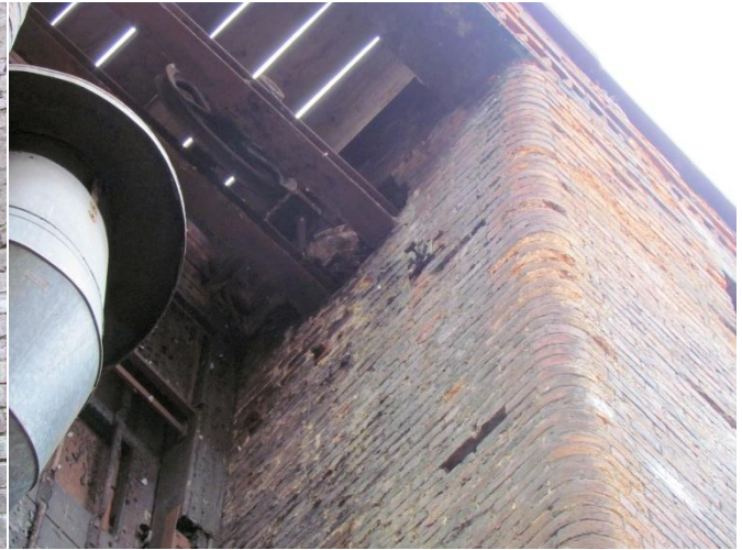
Missing Bricks near Top of Loading Slot
