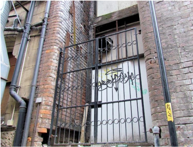
Charred Door Frame and Missing Bricks
