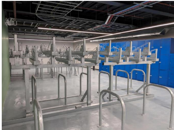
Site Photo: Existing Electric Bike Charge Zone
