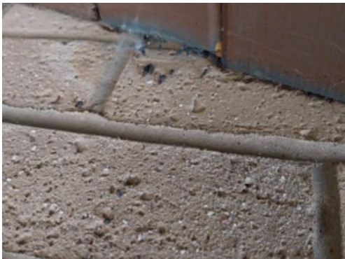
Photograph 13: Gap in roof of B18 with bat droppings
