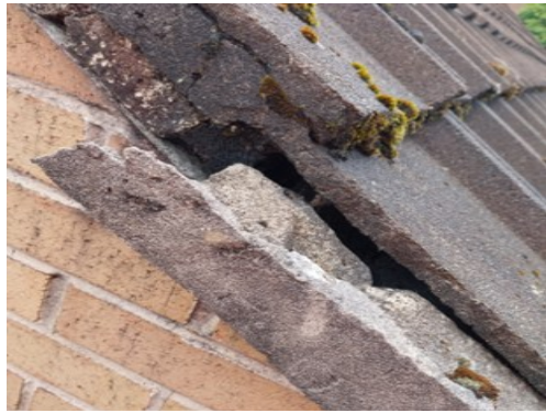
Photograph 10: Gap in slate tile roofing
