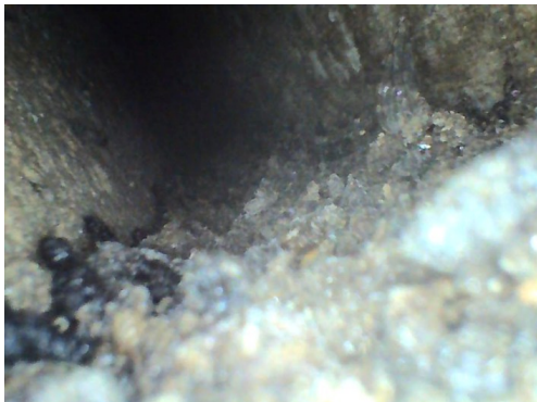
Photograph 21: Endoscope inspection of B18. Bat droppings present
