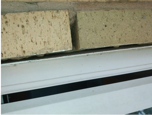
Photograph 3: Missing mortar and weep holes above windows
