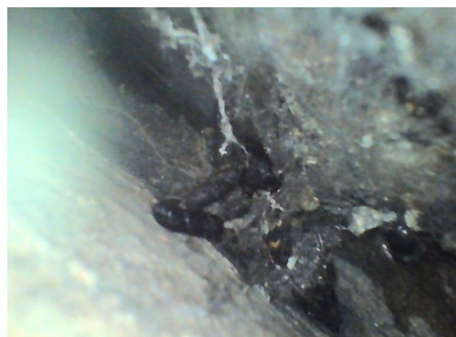
Photograph 24: Endoscope inspection of B18. Bat droppings present
