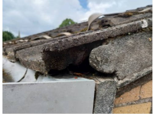
Photograph 4: Gap in slate tile roofing
