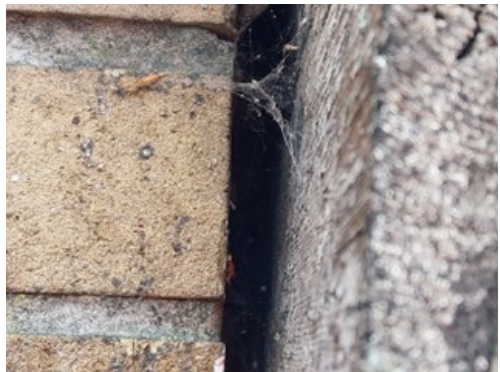
Photograph 6: Gap behind fascia board
