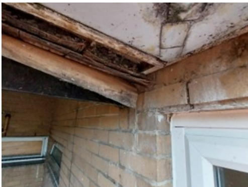
Photograph 7: Rooted wood creating gap in roof
