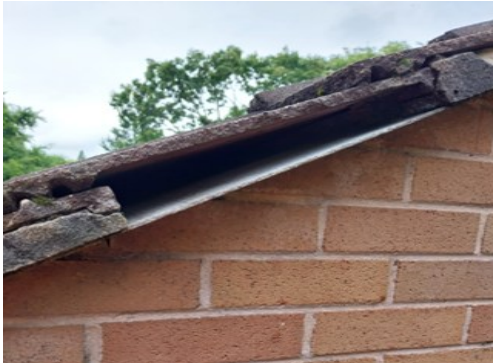
Photograph 11: Gap in slate tile roofing
