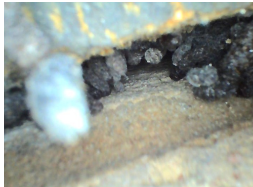
Photograph 22: Endoscope inspection of B19. Bat droppings present
