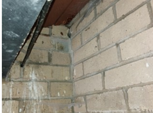
Photograph 12: : Gap in roof of B18 with bat droppings
