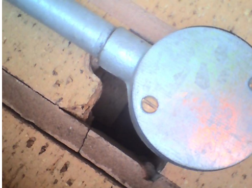
Photograph 19: Gap in wall leading into wall cavity
