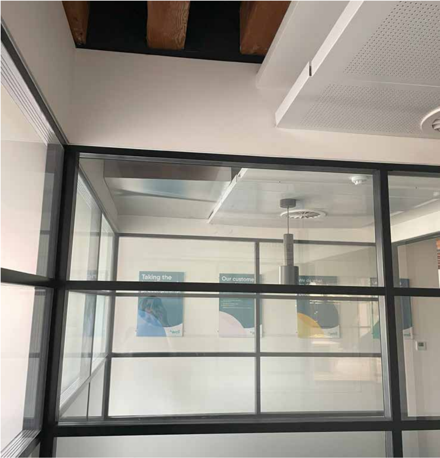
EX.01.04/05 Meeting room - Glazed partition screens, floor boxes and room temperature controllers Dem.01 / 06 / 07 / 08 / 09 / 11
