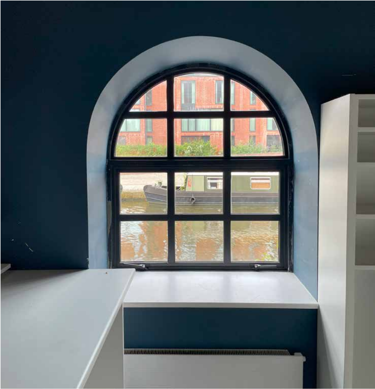
EX.01.06 Private office - Tenant chattels, window condition Dem.01 / 02 / 31
