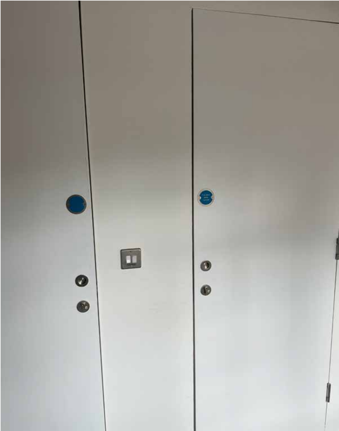
EX.02.14 Store - Riser Doors, floor boxes, glazed partition screen
