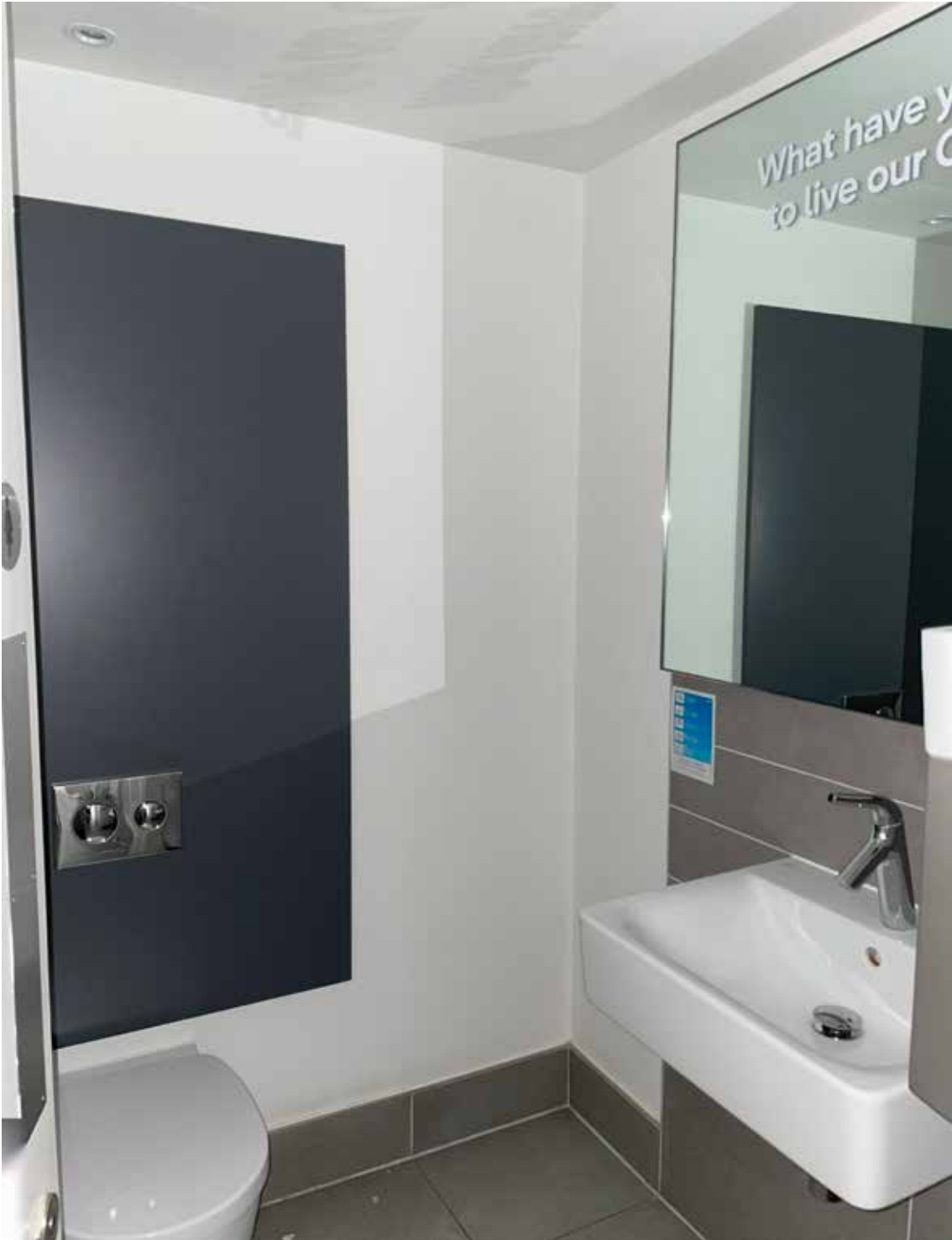
EX.01.27 WC - Signage and fixings Dem.23
