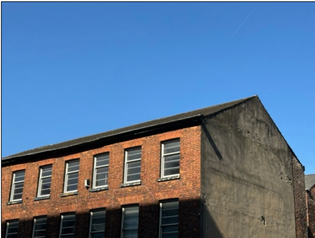
Photograph 6; A wider view of the external roof, which does not highlight many instances of displacement.
