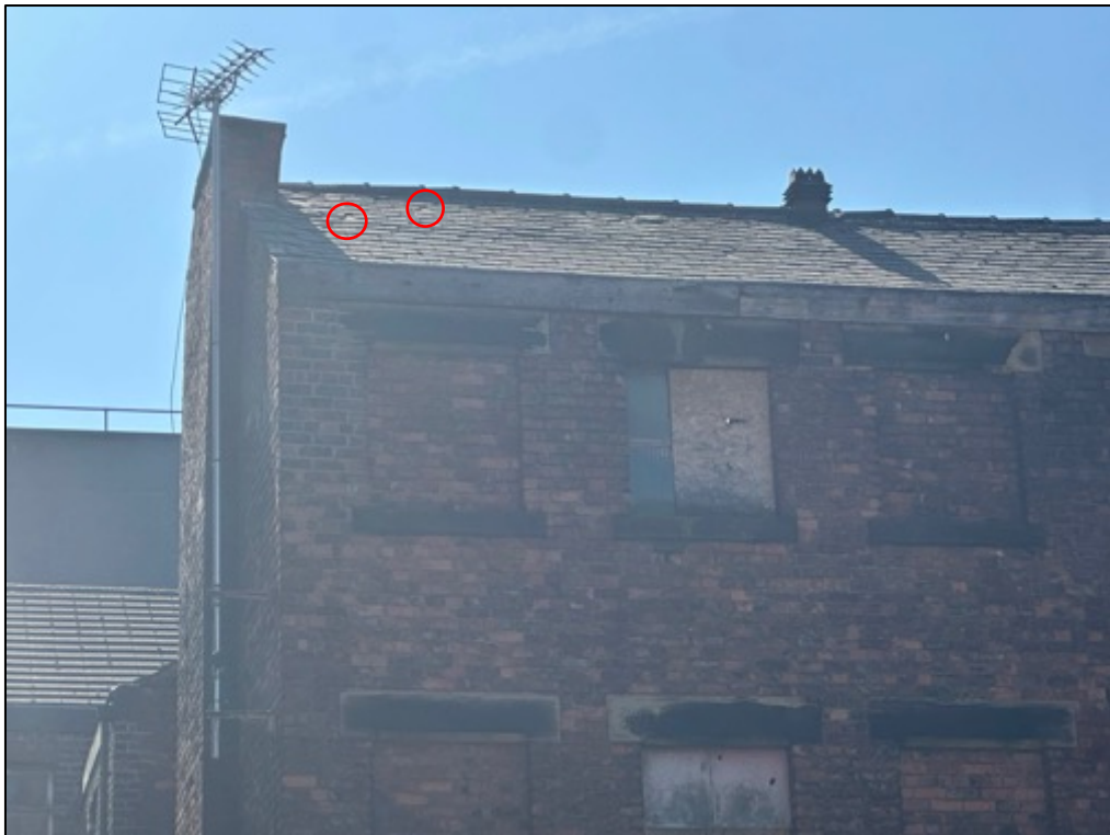
Photograph 2; A closer view of the northern face of the external roof. Some instances of damage/displaced tiles noted across the roof has been circled above.
