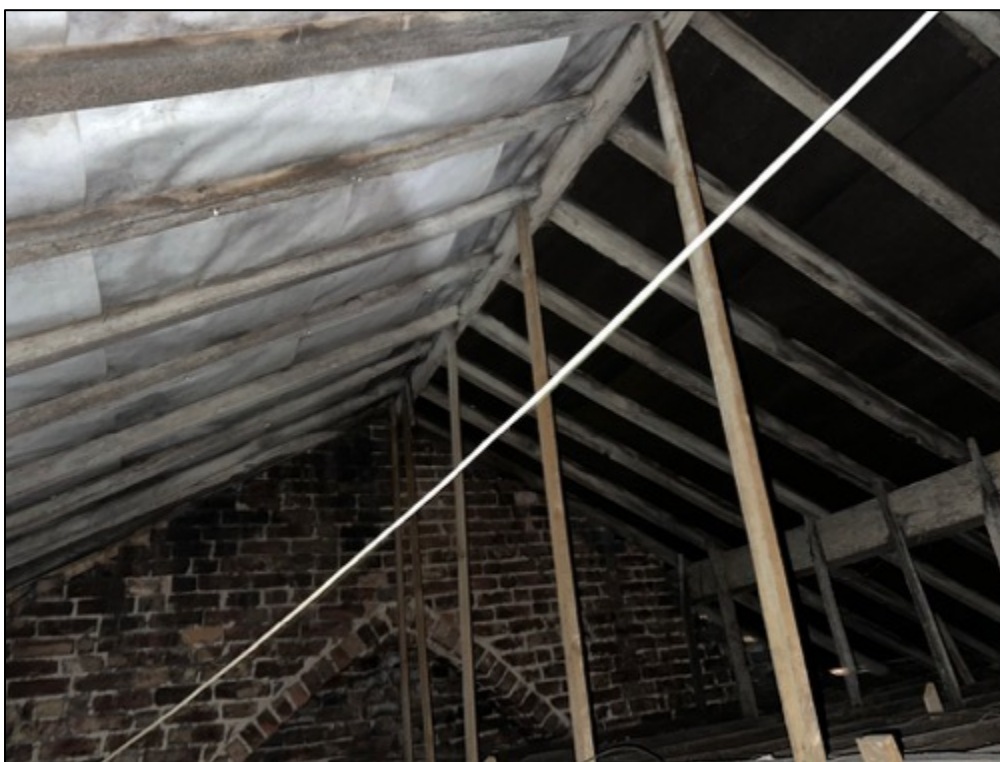
Photograph 8; Another view of the same section of internal roof revealed plastic sheeting installed beneath the external roof covering, with wooden purlins and rafters supporting the roof structure.
