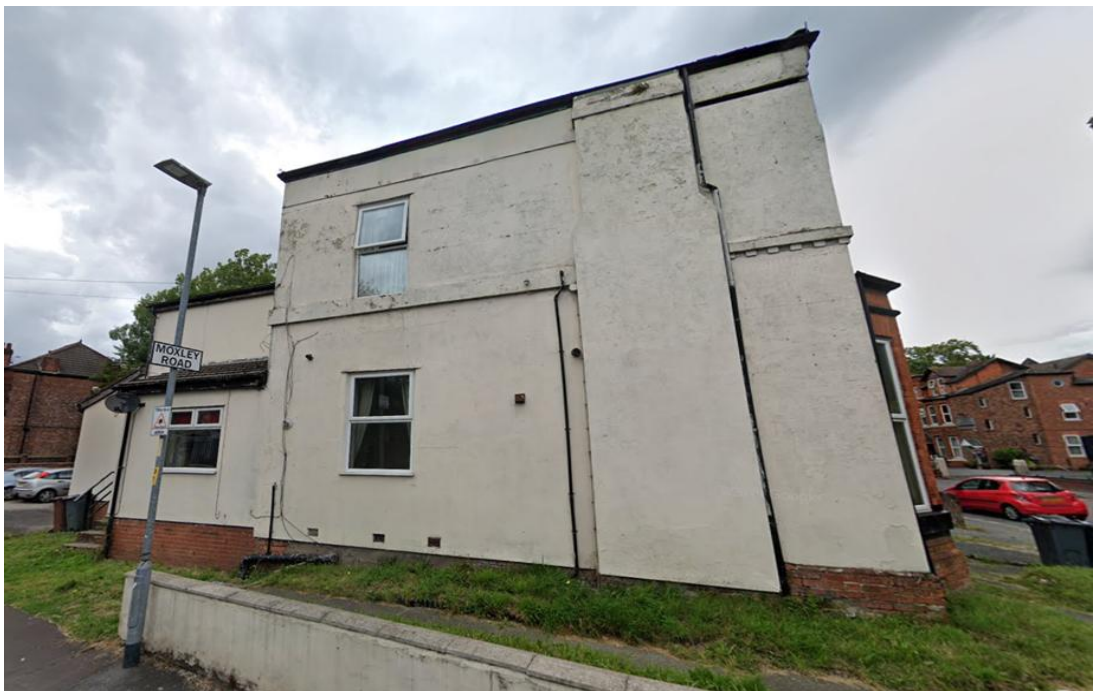
Image 2 – Streetview of side elevation of site from Moxley Road. This view demonstrates poor quality render which obscures the brickwork.
