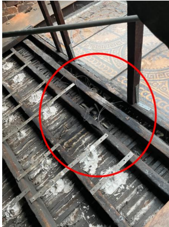
Figure 3.9 Localised water damage near a roof light in the arched section in the N-W corner of the central roof.
