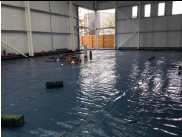
Overview to the membrane line out to unit 1.
