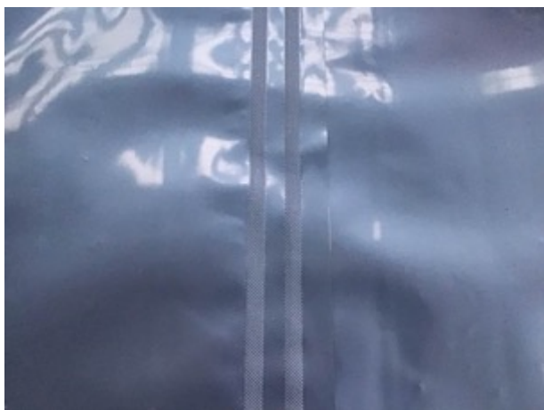
Sealed auto weld
