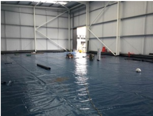
Membrane line out to unit 1
