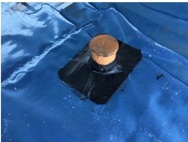
Unit 2 sealed pipe penetration
