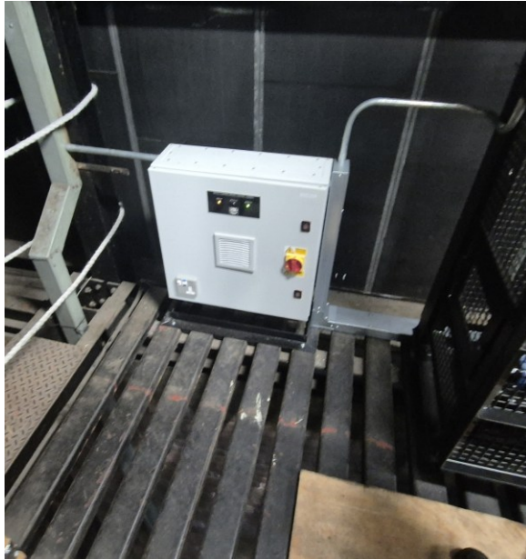
New MCC unit and motorized winch for safety curtain.
