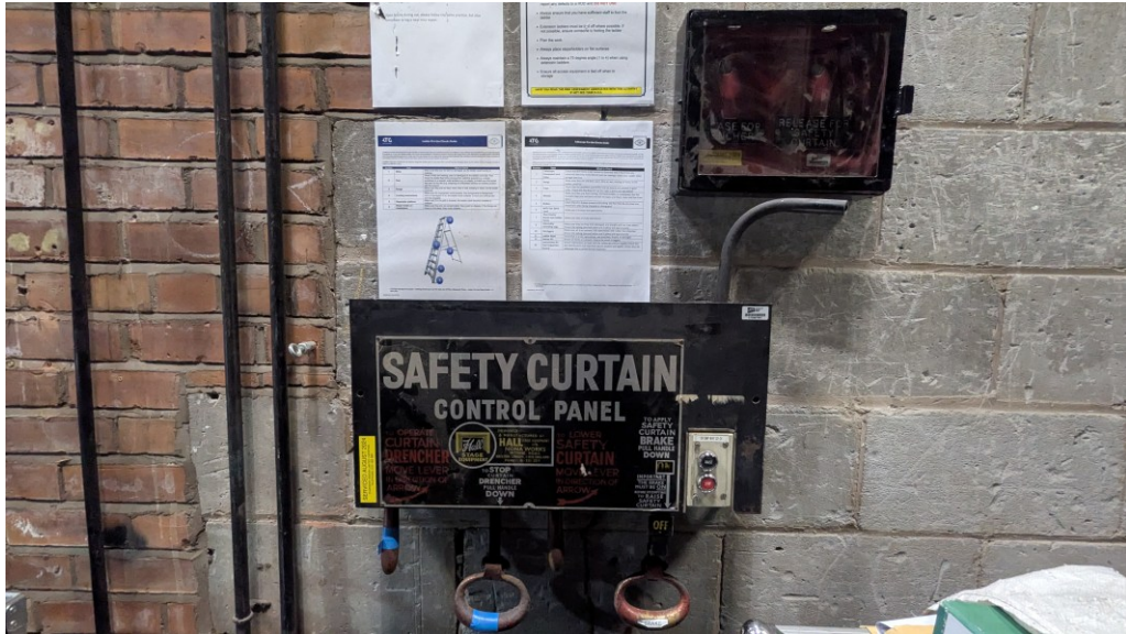
Relocated old safety curtain control panel and release box.
