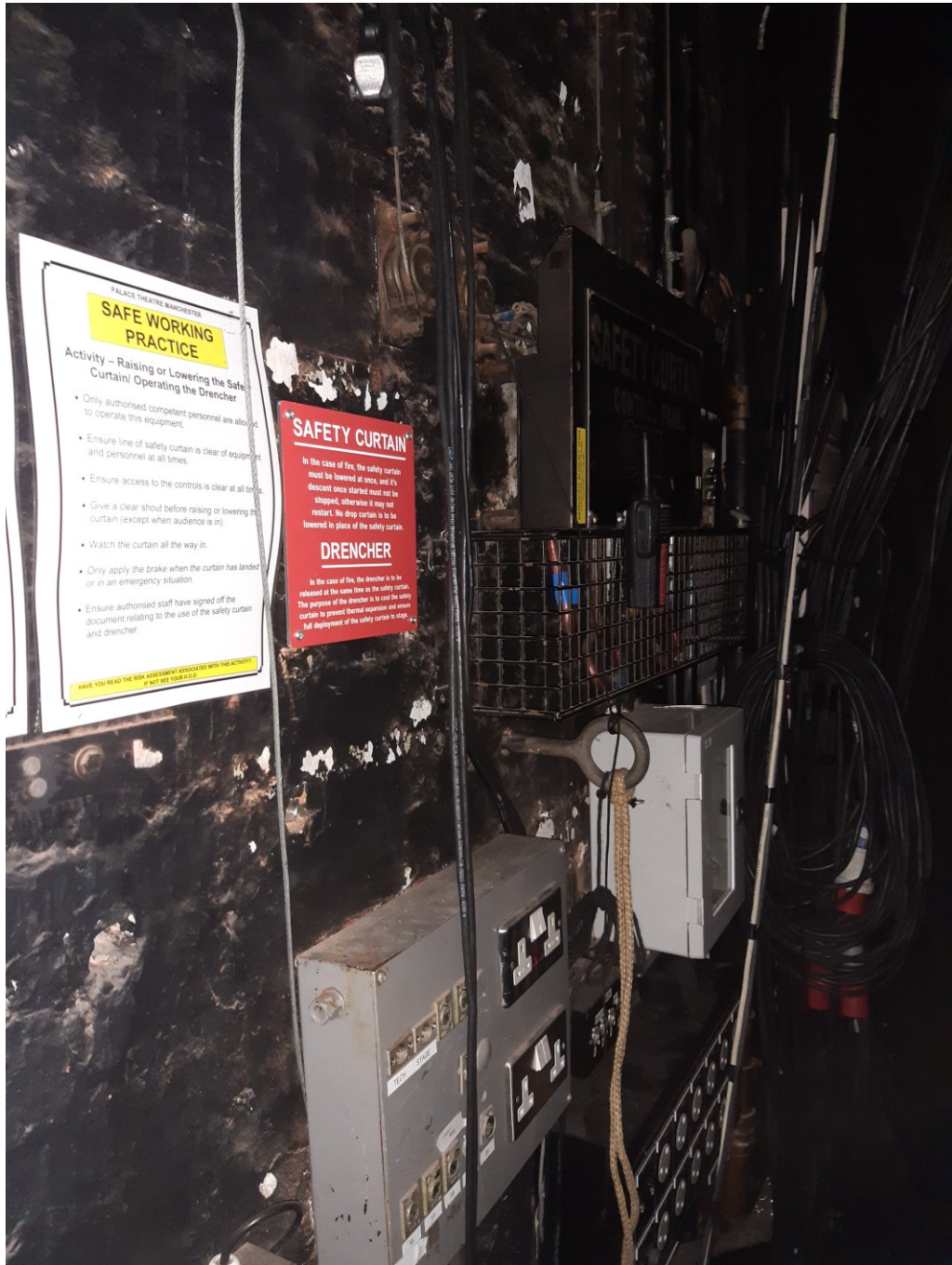
Photo 03 - Existing photograph looking towards the safety curtain control panel and drencher controls stage left.
