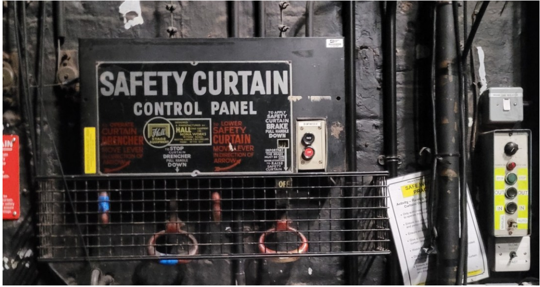
Photo 06 - Existing close-up photograph looking at the existing safety curtain control panel.
