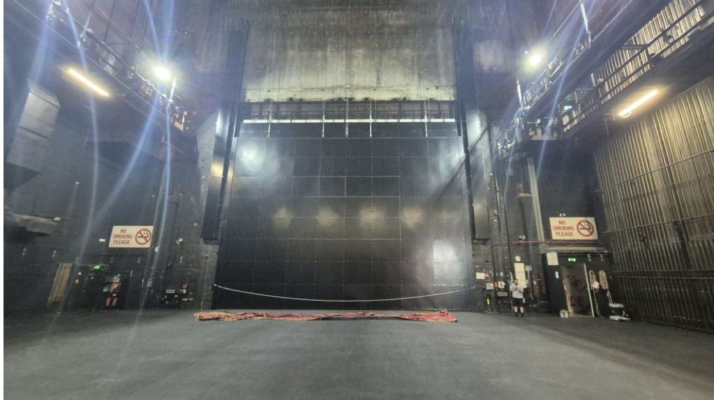
Rear of new safety curtain.
