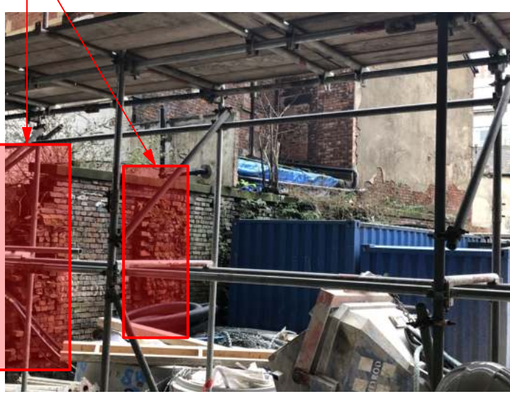
Wall F - Existing condition looks to be in poor condition visually. Key constraint is Booz 4 U boundary
