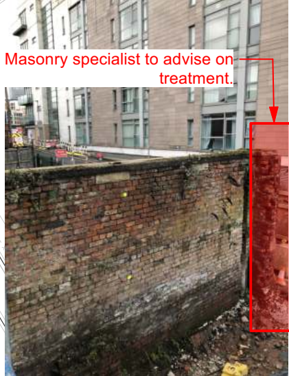
Wall B - Existing condition looks to be in poor condition visually.
