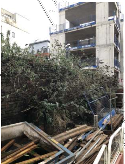
Wall C - Existing condition Looks to be in poor condition with large weeds growing through the structure.
