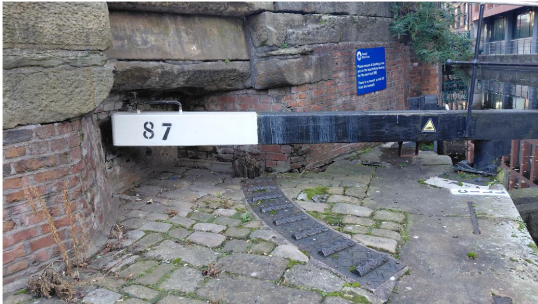
Figure 8 Balance beam of the off-side top gate creates a trapping hazard against the wall
