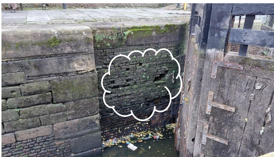
Figure 5 Missing brickwork (towpath side gate recess) to be repaired
