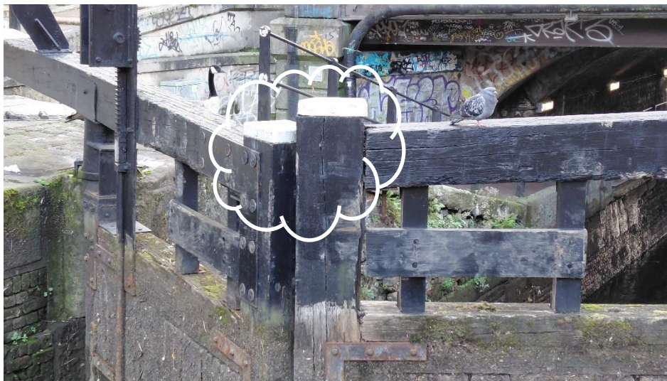
Figure 2 Bottom gates (condition)
