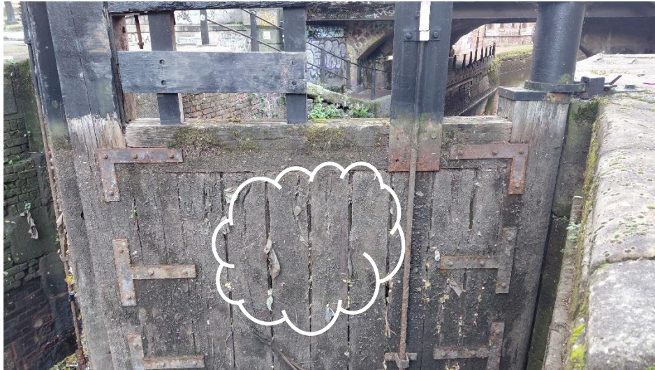
Figure 3 Bottom gates (condition)
