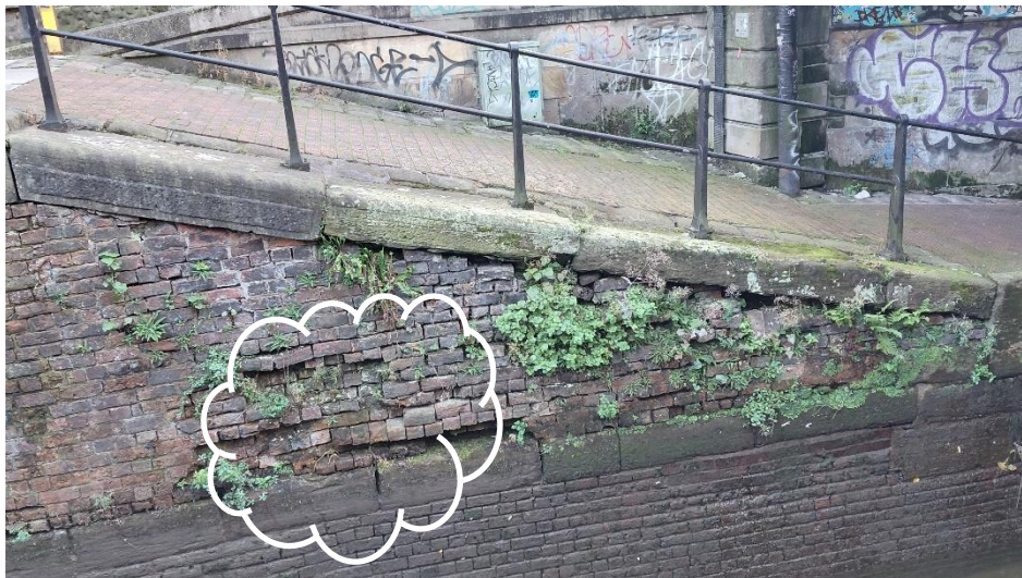
Figure 4 Missing and unstable brickwork (towpath side forebay) to be repaired
