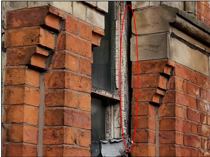
Photograph 6 showing the gap in masonry on the southwest elevation
