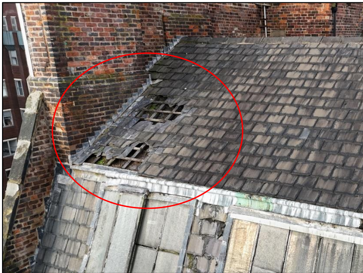
Photograph 3 showing the missing tiles
