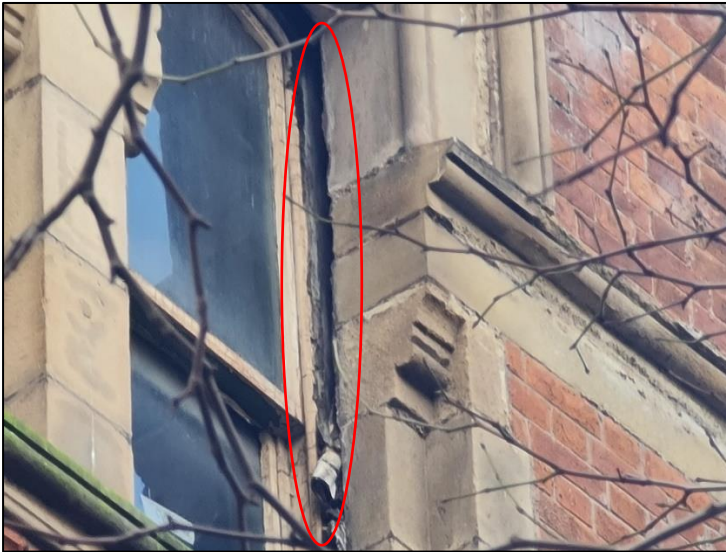
Photograph 5 showing the gap in masonry on the northeast elevation
