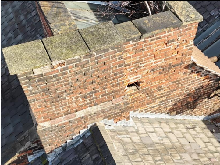
Photograph 4 showing the gap in the brickwork
