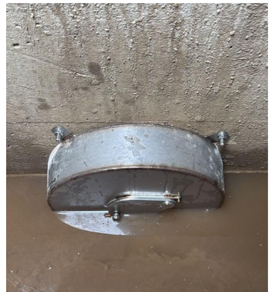
Photo. 08 – As fitted flow control
