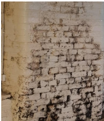
C - Internal Masonry Wall Exposed existing brickwork,. Surface discoloration may be due to trapped moisture, potentially caused by non-breathable paint preventing proper evaporation.
