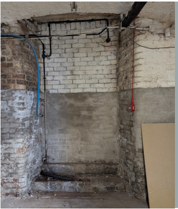
D - Brick infilled fire escape This area shows a former fire escape that has been infilled with brick,
