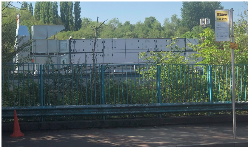
Figure 1, AHU seen on site, photo dated 30 April 2025.
