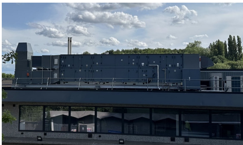
Figure 2, Finished AHU and ductwork wrapped in vinyl (photo from agent, photo received 2 July 2025)
