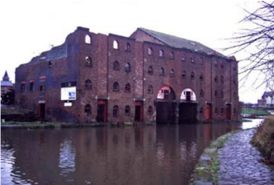
1995 Deteriorated condition - west and north elevation
