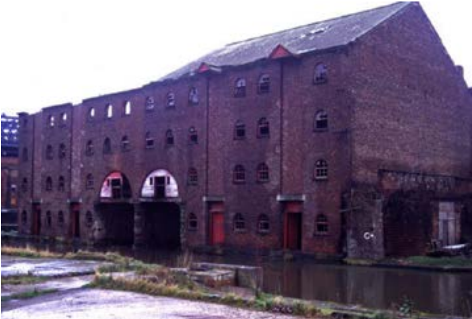
1995 Deteriorated condition - west and south elevations
