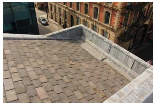
Roof – the low parapets pose a risk when attempting to clean lead gutters
