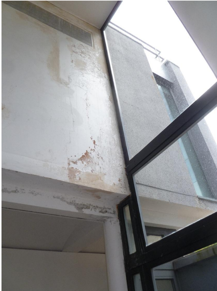
Figure 3.1: Internal damp evidences the failing building envelope of Prospect House
