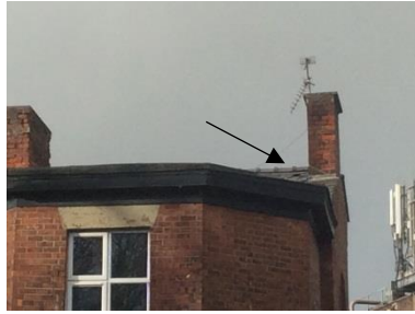
B2; Slipped roof slate
