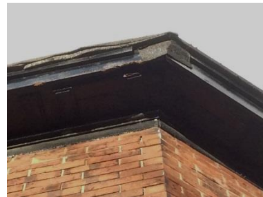
B2; Lifted felt above soffit box
