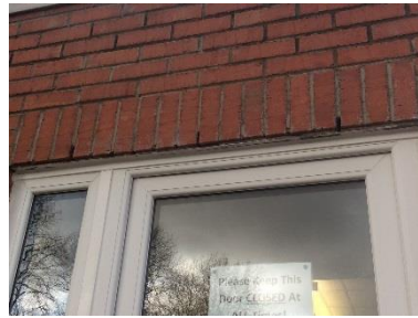
B1; gaps in the mortar
