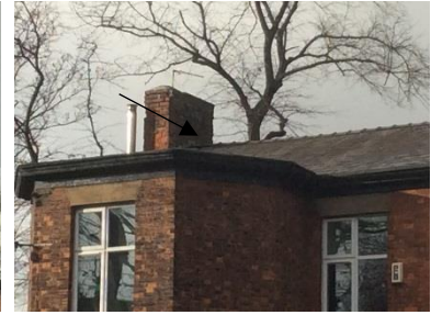
B2; Lifted ridge roof slate
