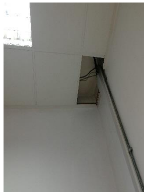
B2; Missing tile revealing roof
