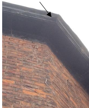
B2; Large hole in soffit box
