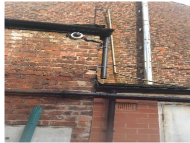
B2a; Lifted roof felt
