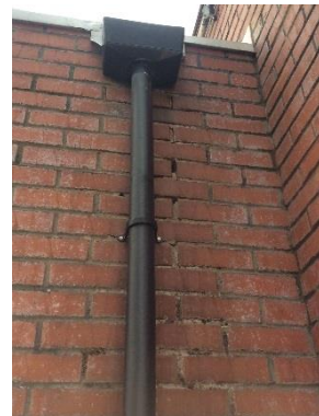
B1; gaps in the mortar
