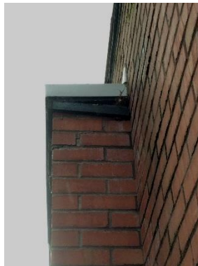
B1; gap behind bargeboard
