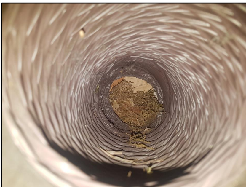
Photograph 3 showing the vent
