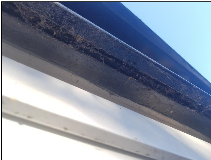
Photograph 2 showing the gap between the cladding and the window
